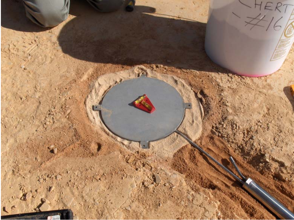
Figure 3-14: Geokon Model 3500 Earth Pressure Cell at the Test Track.
