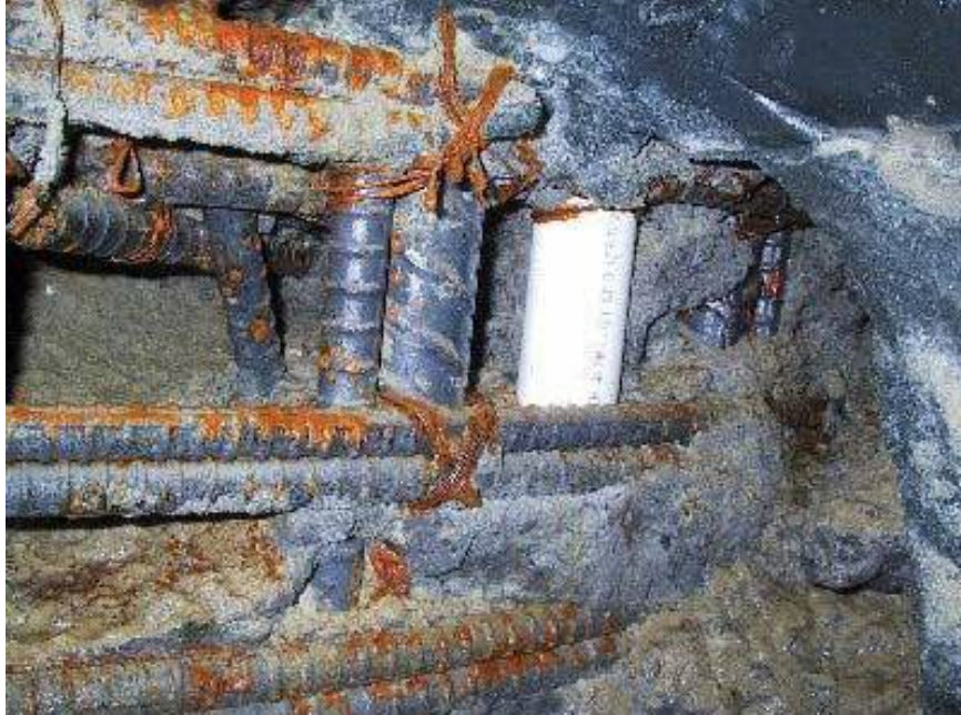
Figure 2.31: Shaft defect due to congested reinforcement cage (Bailey 2005)
