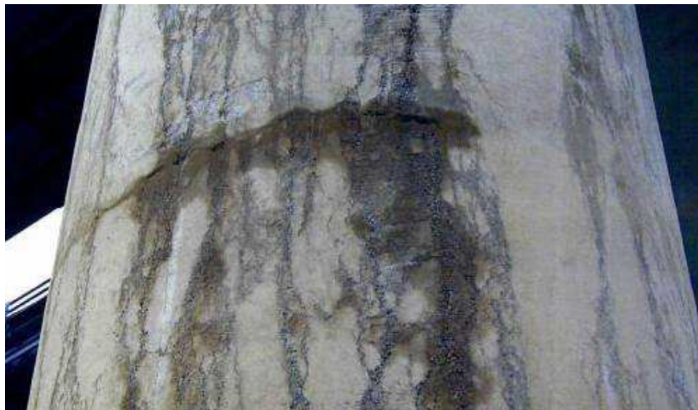
Figure 2.33: Bleed water channels of exposed surface of drilled shaft (Brown and Schindler 2007)
