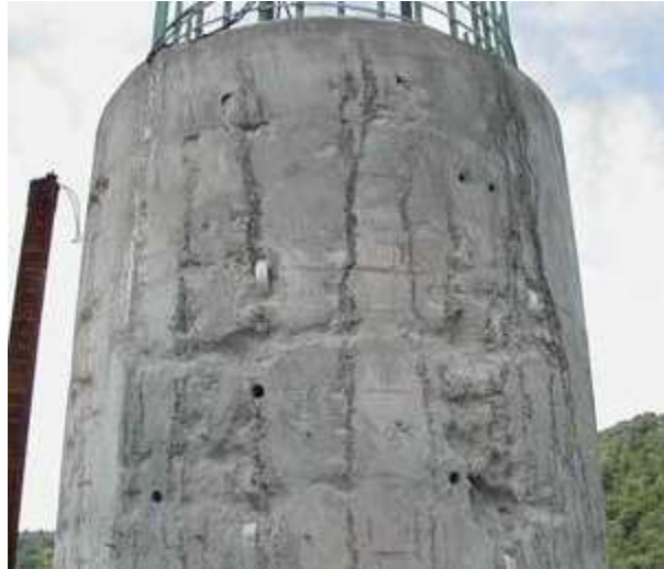
Figure 2.27: Entrapped laitance found after casing removal (Brown and Schindler 2006)
