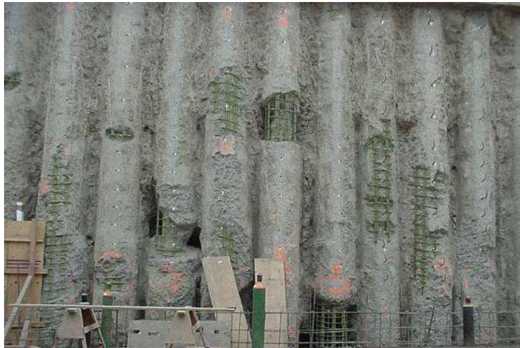
Figure 2.24: Shaft defects due to improper workability (Brown 2006)
