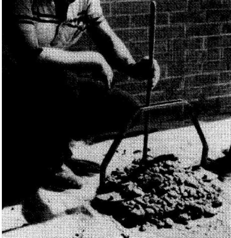
Figure 2.20: Concrete with adequate workability but large aggregate for tremie placement (O'Neill and Reese 1999)
