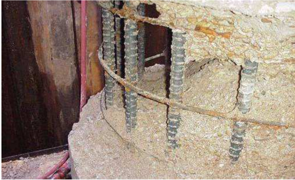
Figure 2.23: Shaft defects due to improper workability (Bailey 2005)
