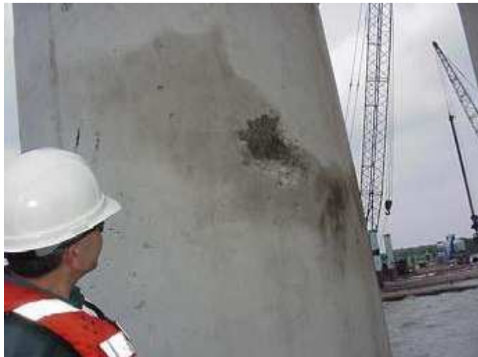
Figure 2.26: Entrapped laitance found after casing removal (Brown and Schindler 2006)
