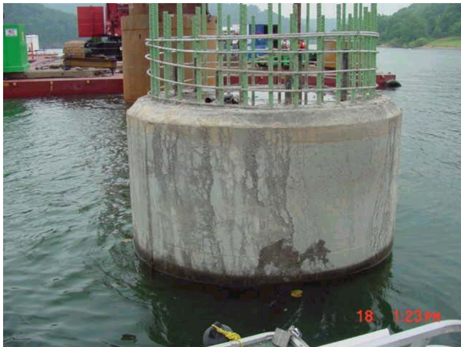
Figure 3.24 – Example 1 of Bleed Channels and Surface Streaks due to Bleed Water Traveling along the Casing (photograph courtesy of Dr. Dan Brown)
