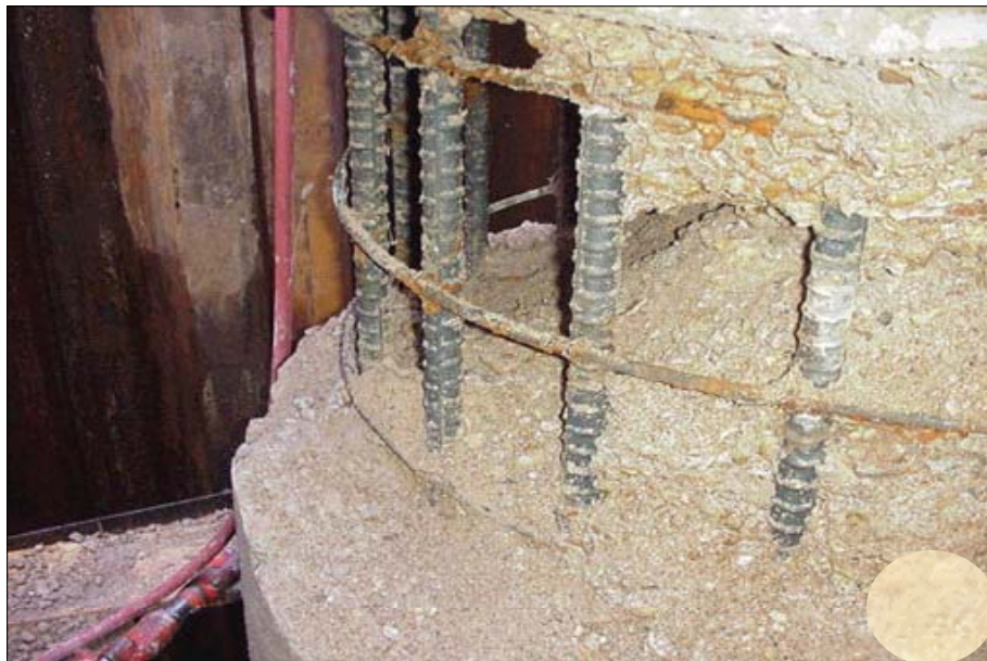
Figure 3.7 - Example 2 of Shaft Defects due to the Loss of Workability (TxDOT)
