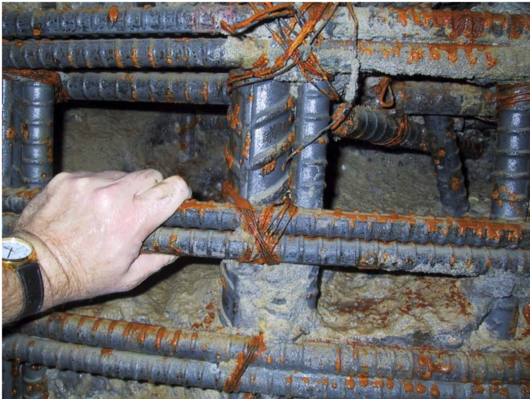
Figure 3.22 – Shaft Defect due to Double Reinforcement Cages (photograph courtesy of Dr. Dan Brown)
