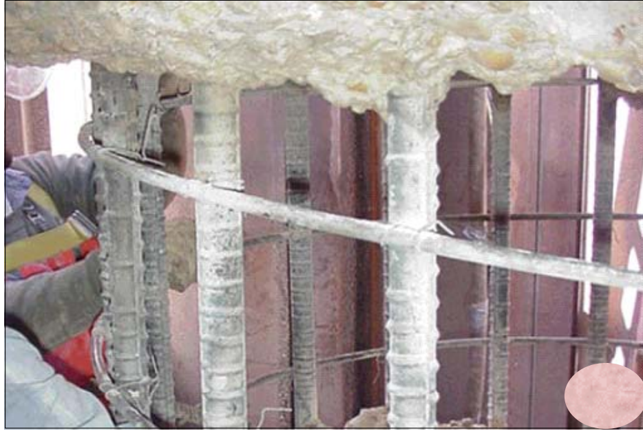
Figure 3.10 - Example 5 of Shaft Defects due to the Loss of Workability (TxDOT)
