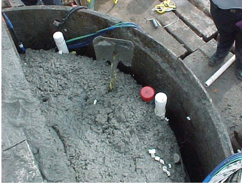
Figure 3.19 - Elevation Difference between the Inside and Outside of a Rebar Cage due to Screening of the Concrete Flow (photograph courtesy of Dr. Dan Brown)
