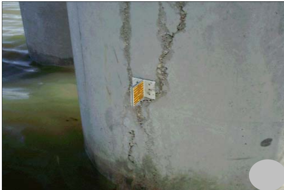
Figure 3.26 - Shaft Defect due to Bleed Water Traveling along the Casing (TxDOT)
