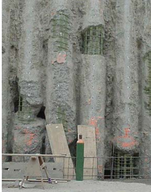
Figure 3.6 - Example 1 of Shaft Defects due to the Loss of Workability (photograph courtesy of Dr. Dan Brown)
