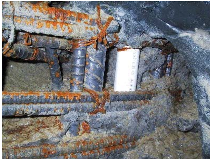
Figure 3.20 – Shaft Defects due to the Screening of the Concrete Flow (photograph courtesy of Dr. Dan Brown)
