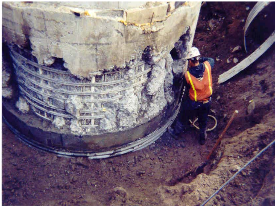
Figure 3.9 - Example 4 of Shaft Defects due to the Loss of Workability (Caltrans)
