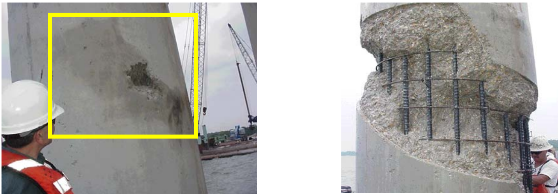
Figure 3.16 - Shaft Defects due to the Loss of Workability (left), After Removal of Surface Flaws for Repairs (photograph courtesy of Dr. Dan Brown)
