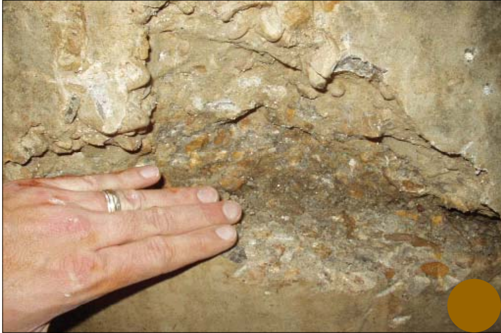
Figure 3.8 - Example 3 of Shaft Defects due to the Loss of Workability (TxDOT)
