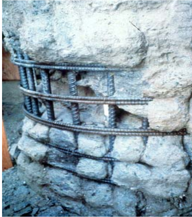
Figure 3.17 - Shaft Defects due to the Loss of Workability from Construction Delays (O'Neill and Reese 1999)
