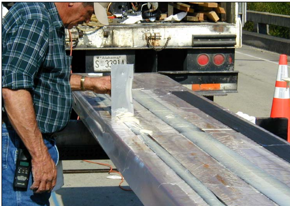
Figure 4.7: Application of Tyfo TC Epoxy to the Composite Strip
