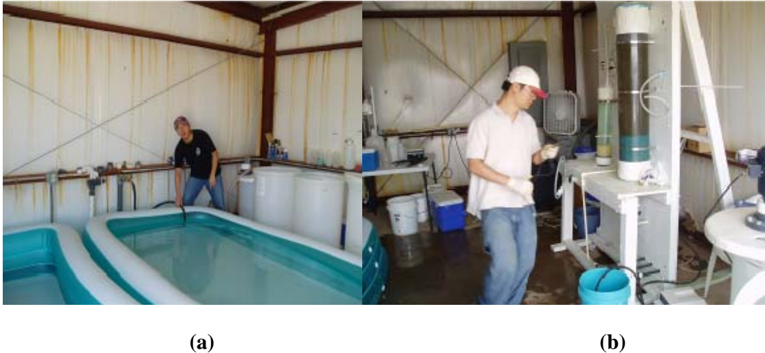
Figure 5-3. Raw water equalizing tanks (the swimming pools) (a) and the pilot test column set-up (b) at the pilot testing site, Well 303, EPWU.
