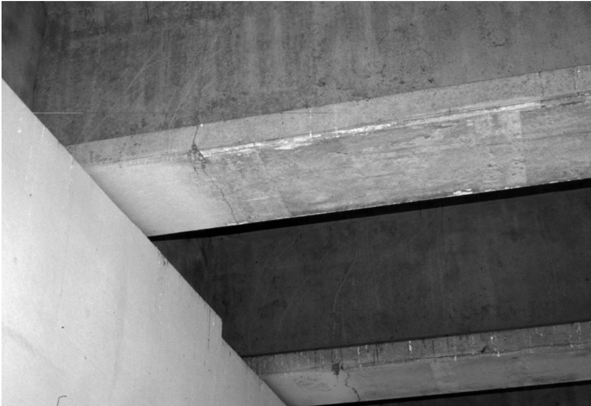
Figure 2-1: Cracks in Continuous Ends of Girders (Barnes 2007)
