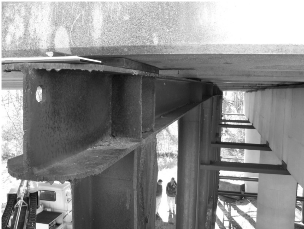
Figure 2-5: Bearing Pad Between Top of False Support and Bottom of Bulb-Tee Girder
