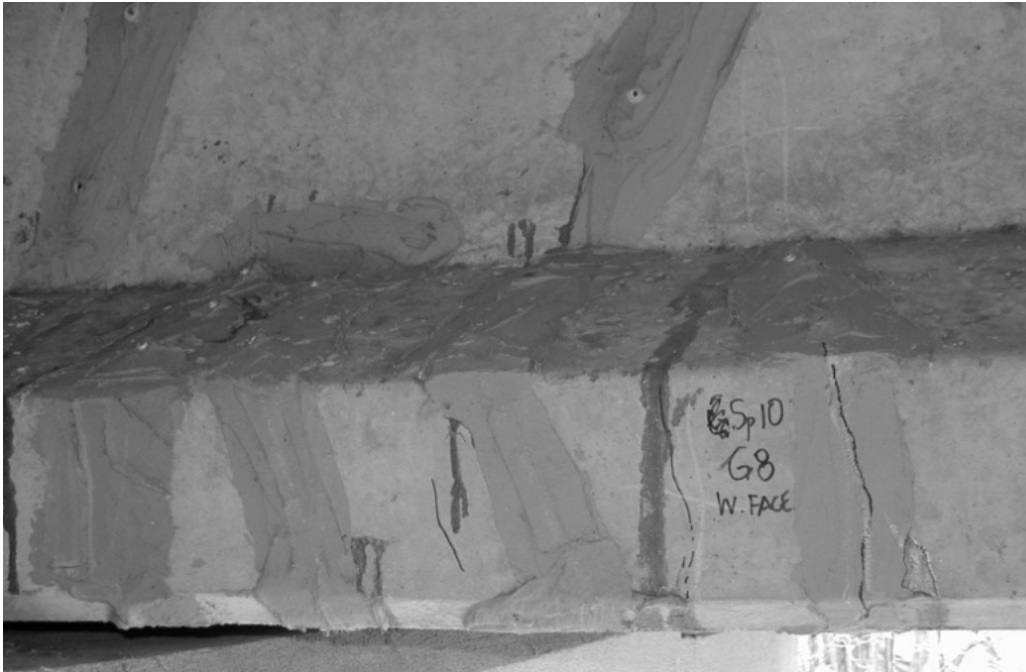
Figure 3-6: Epoxy Sealant to be Removed from Girders Prior to FRP Installation.
