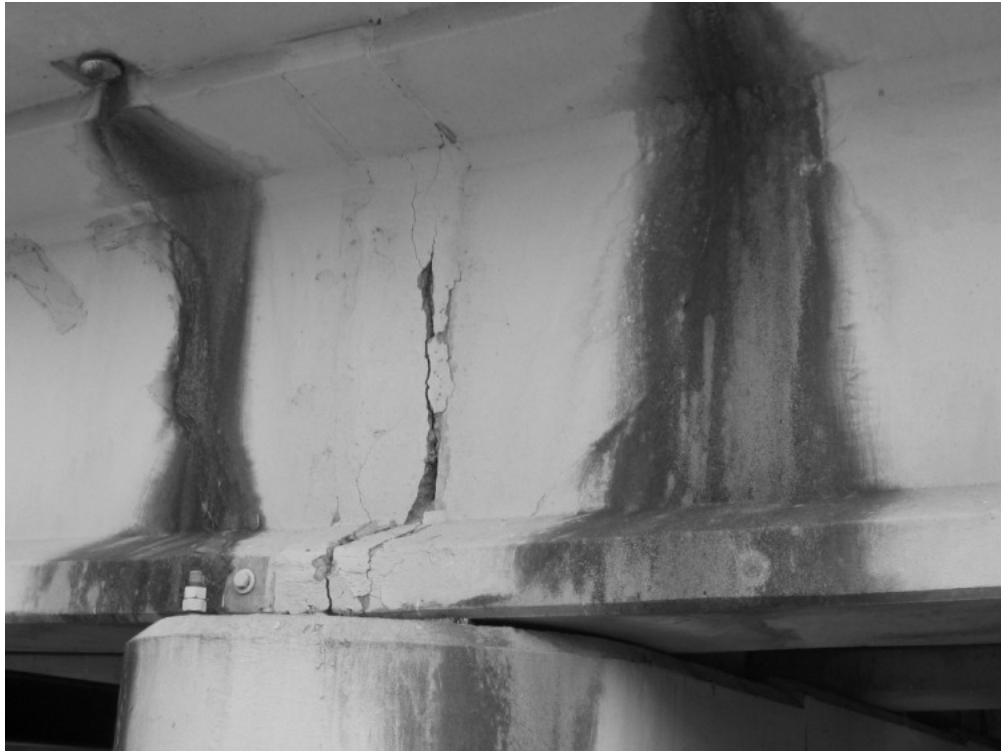
Figure 2-3: End Cracks in the Continuity Diaphragm
