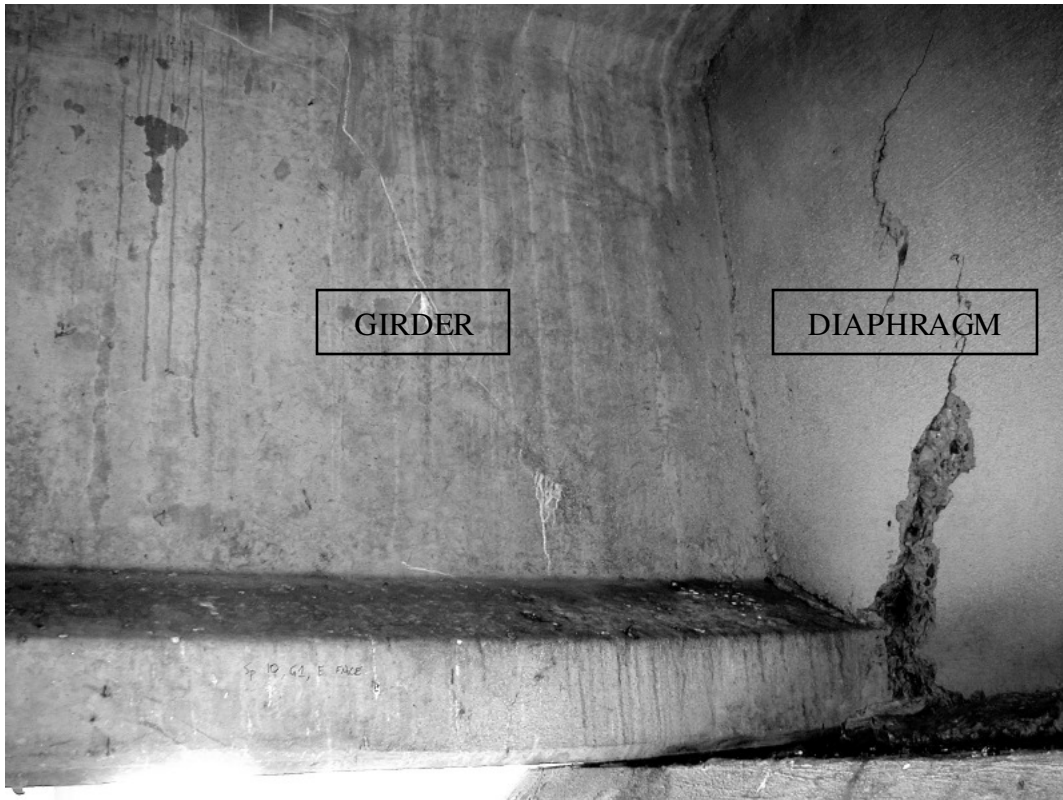
Figure 2-2: Cracks in Continuity Diaphragm
