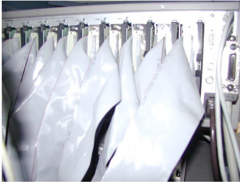
Figure 15 - Multiplexer Cards with Ribbon Cables [19]
