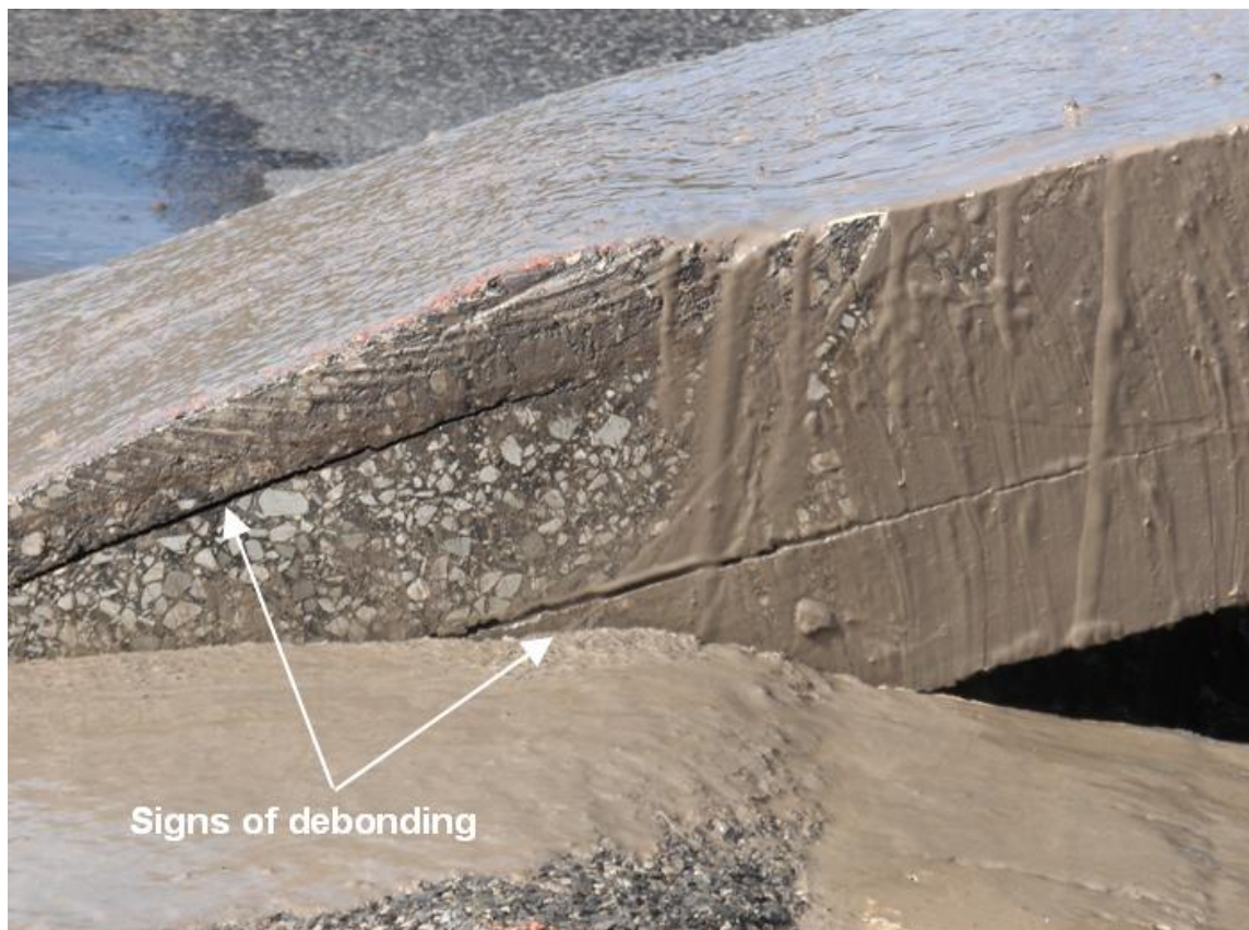
Figure 4. 13 Trench Showing Signs of Debonding in Section N10.
