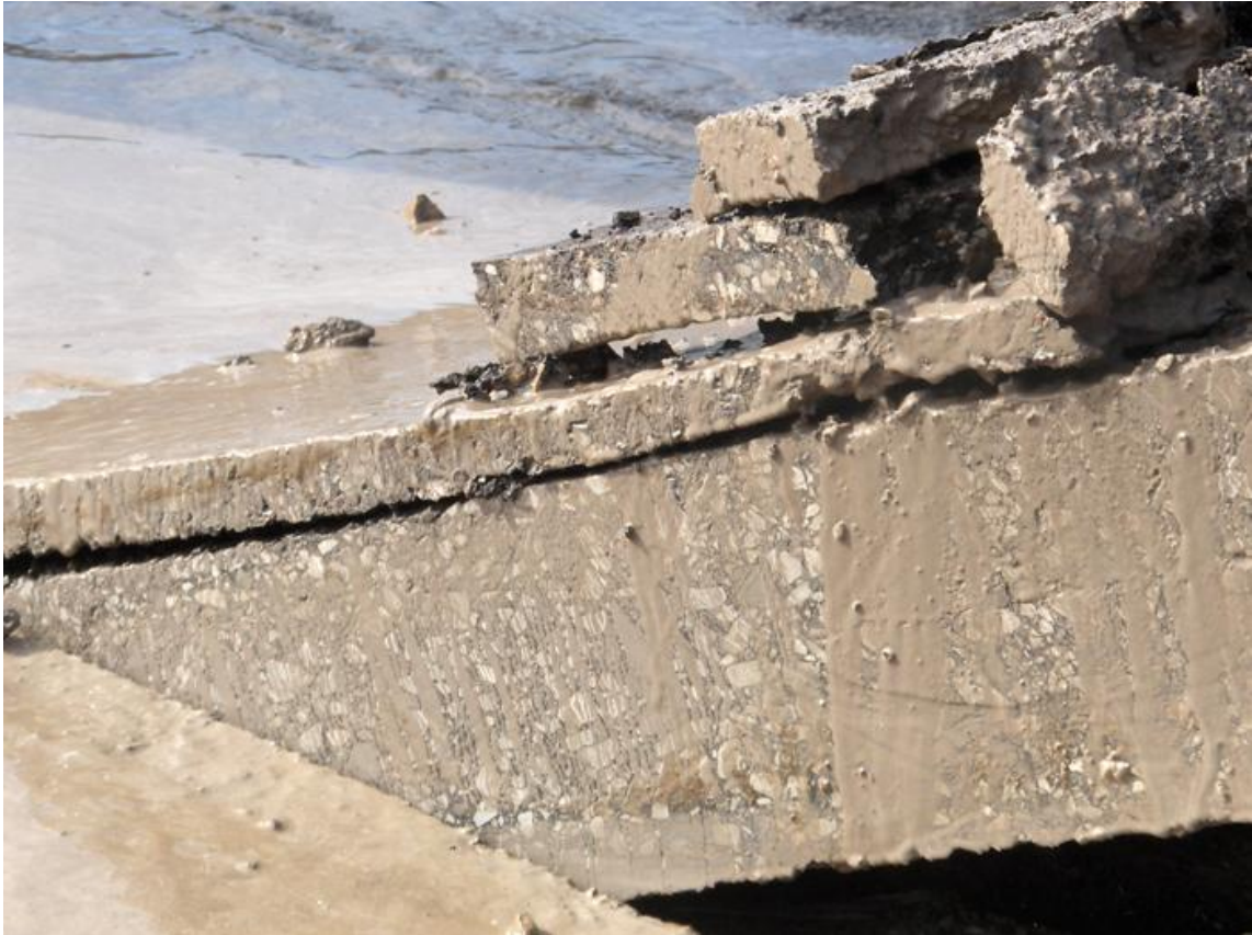
Figure 4. 14 Trench Showing Delamination of HMA Lifts in Section N10.
