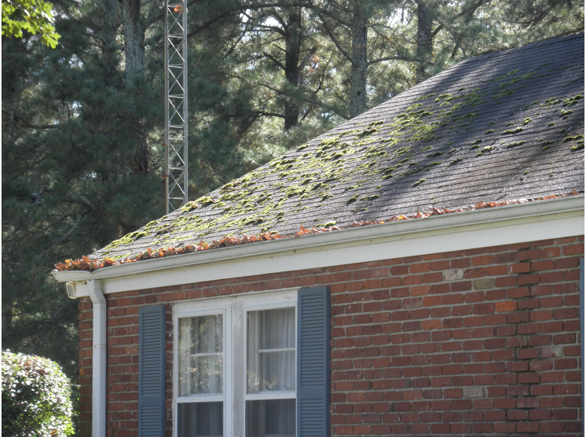
FIGURE 30: Moss and Mold Growing on the North-Facing Roof
