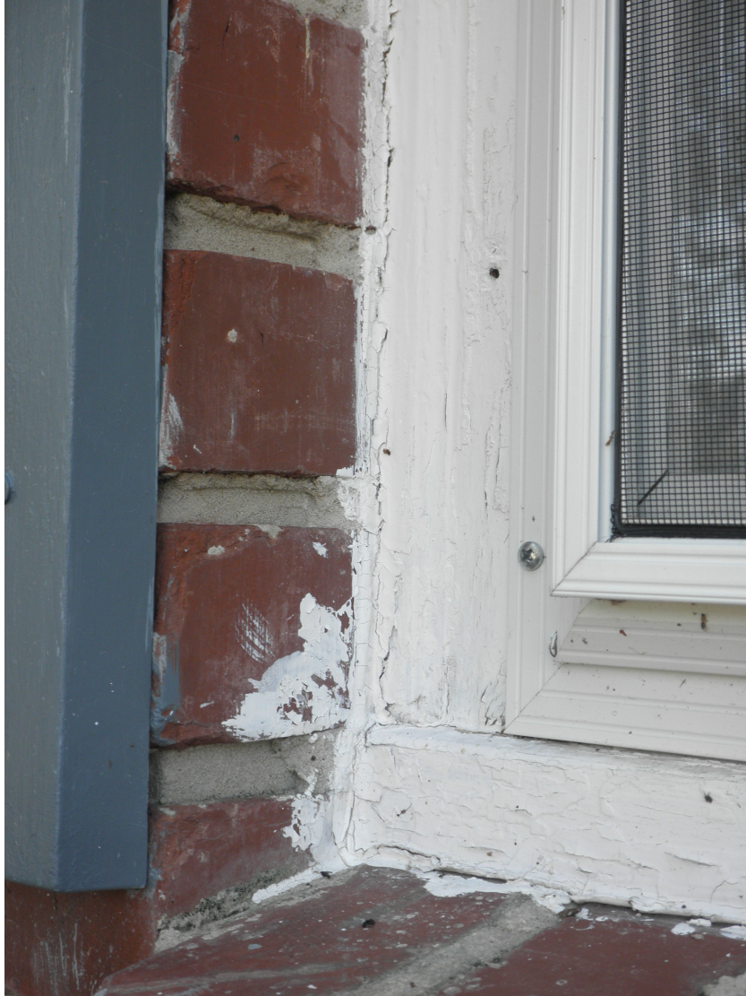
FIGURE 25: Caulk in Need of Replacement
