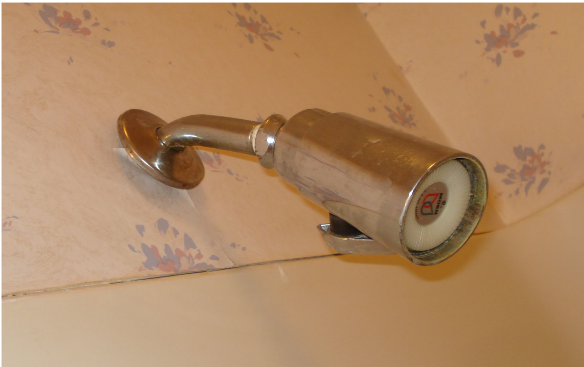
FIGURE 36: Shower Head in Need of Replacement
