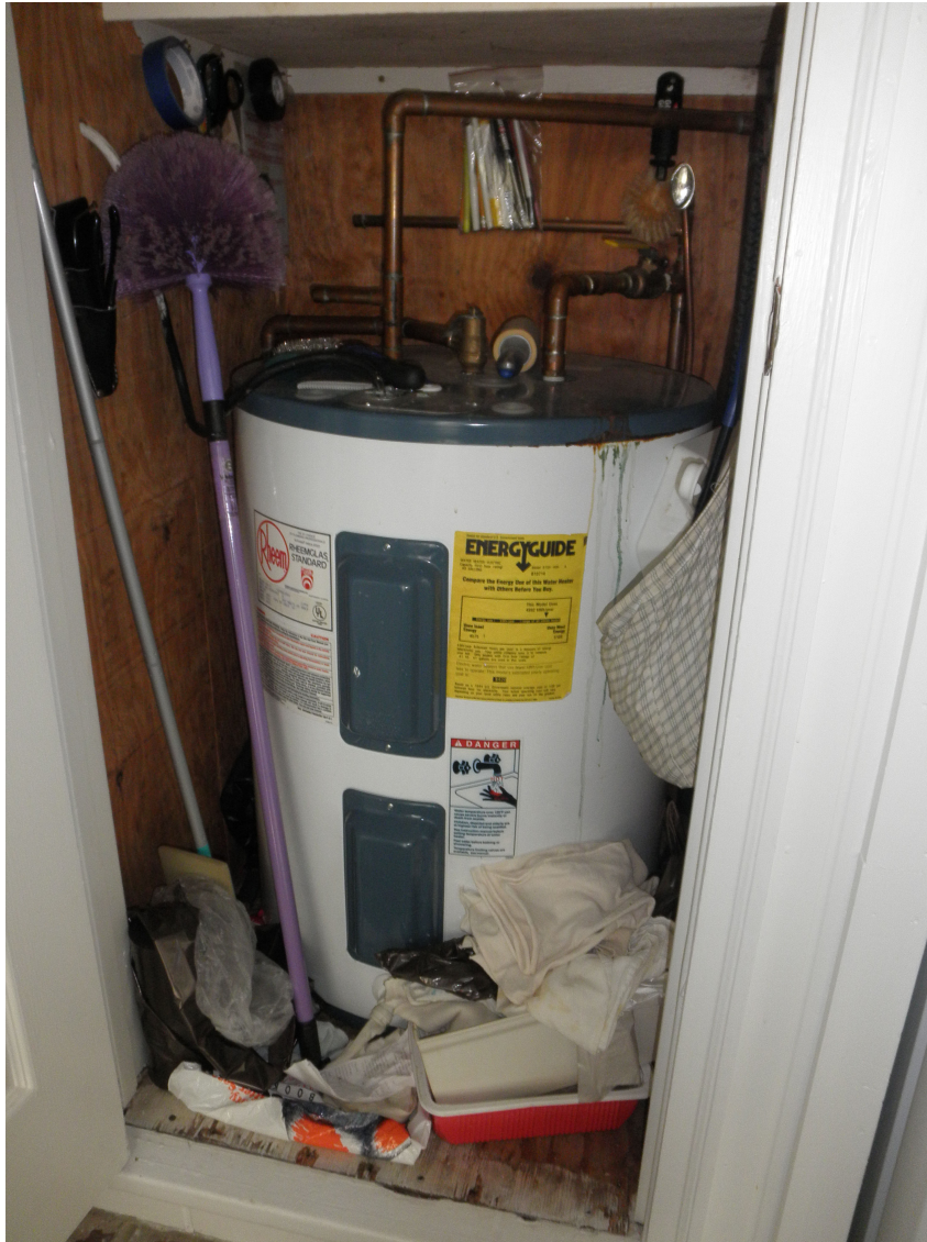
FIGURE 35: Hot Water Heater
