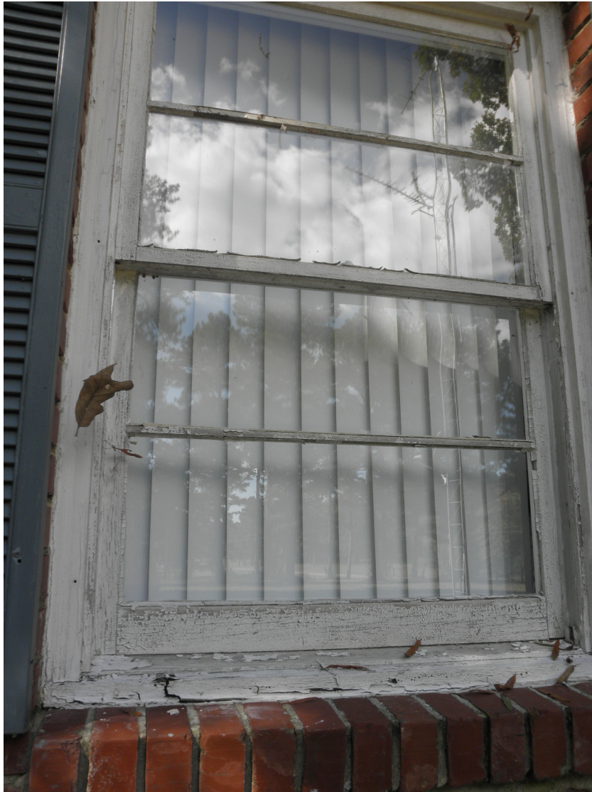
FIGURE 26: Window in Need of Replacement
