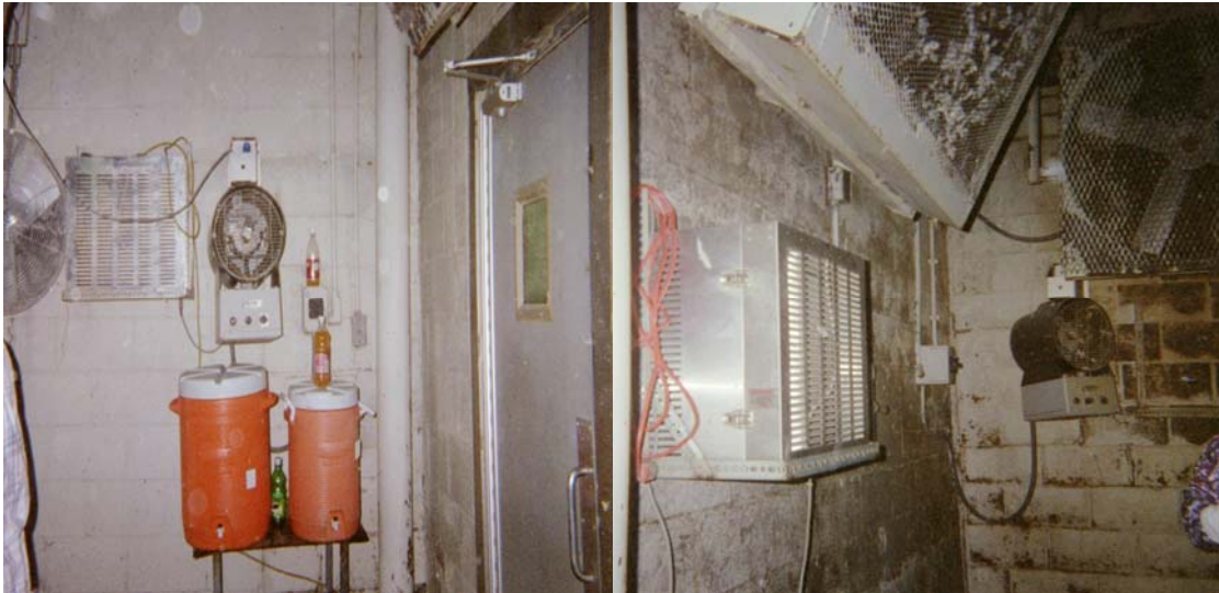
Figure 2: Position 1. Filter was positioned beside a fan, directly to the right of the first hang crew worker.
