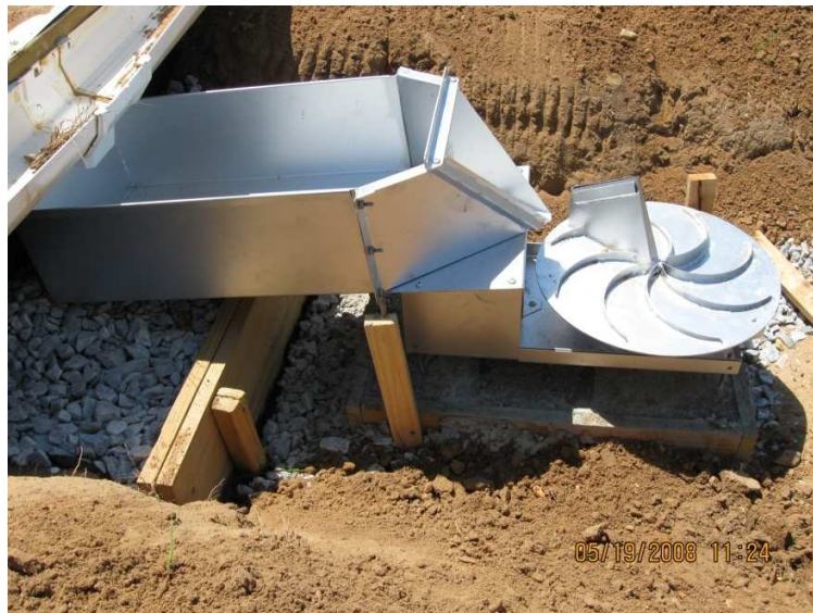
Figure 7: Fabricated Coshocton wheel installed at test plots. Top figure courtesy of Bonta (2002).
