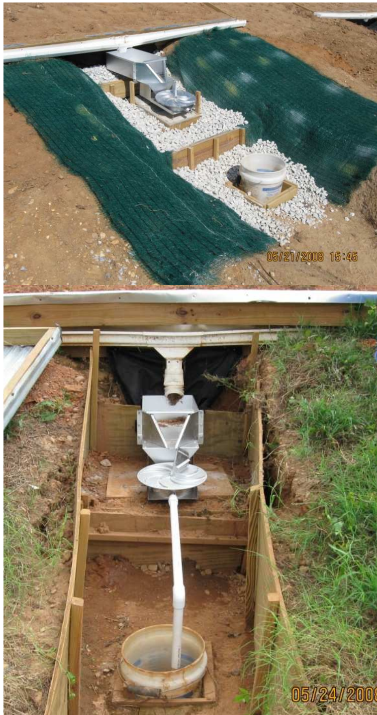
Figure 6: Proportional Coshocton wheel sampler installed with runoff downspout in excavated trench at E.V.Smith.
