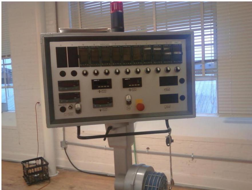
Figure 4.5 Control panel of the twin screw extruder
