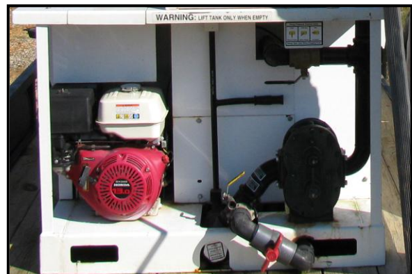
(c) Engine and Discharge Pump
