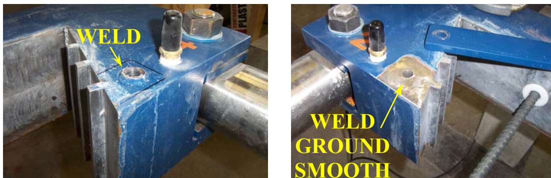
Figure 4-9: Crosshead before and after grinding
