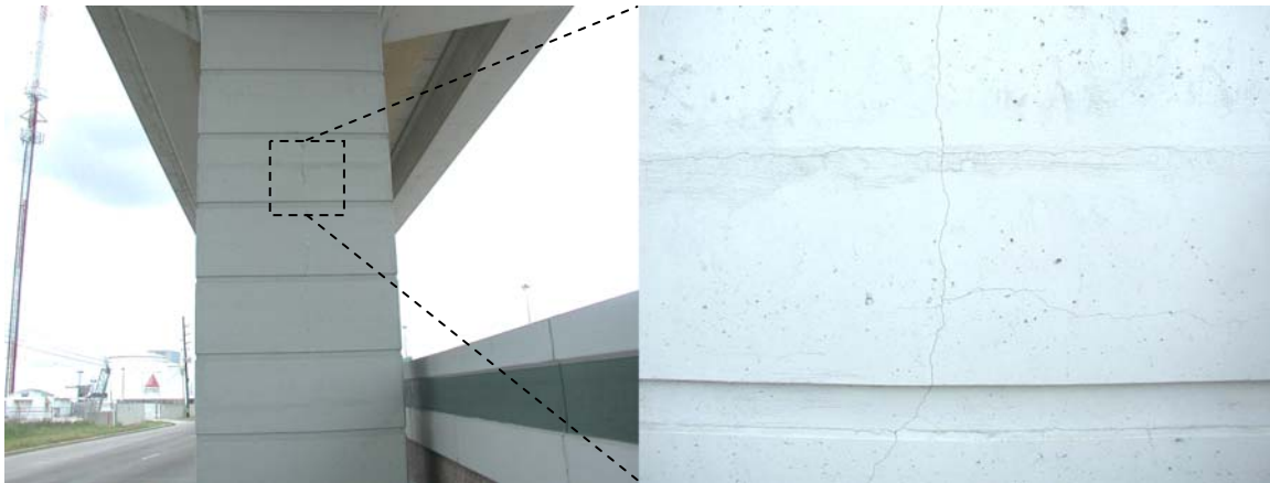
Figure 1-1: Mass concrete cracking in the IH 45/BW 8 interchange, Houston TX
