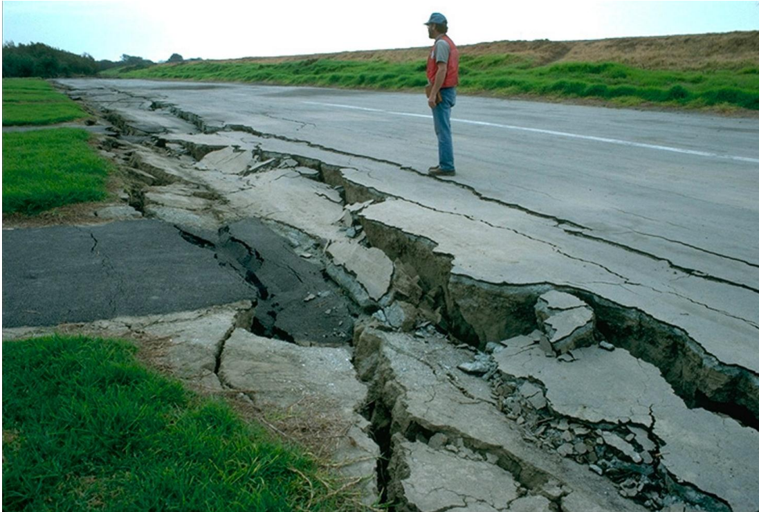
Figure 2.1: Lateral spread roadway failure caused by the Oct. 17, 1989, Loma Prieta earthquake in California (NASA 2010)
