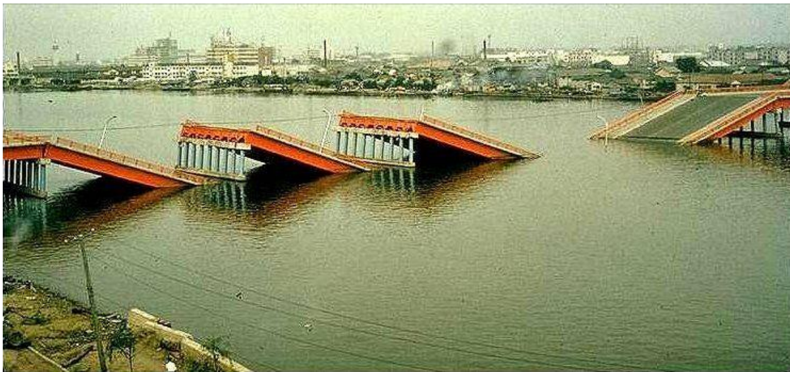
Figure 2.6: Shaw bridge failure caused by lateral spread of the foundation soils after the 1964 Niigata, Japan, earthquake (Johnson 2000a)
