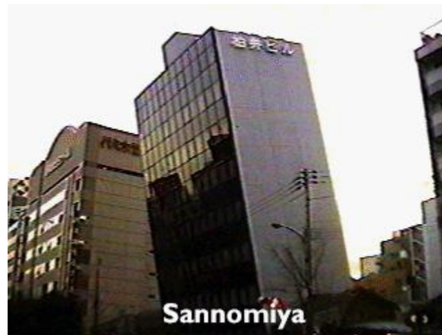
Figure 2.9: Partial bearing capacity failure of a building founded on liquefiable soil in Kobe, Japan, after the 1995 Hyogo-Ken Nanbu Earthquake (Louie 1996)
