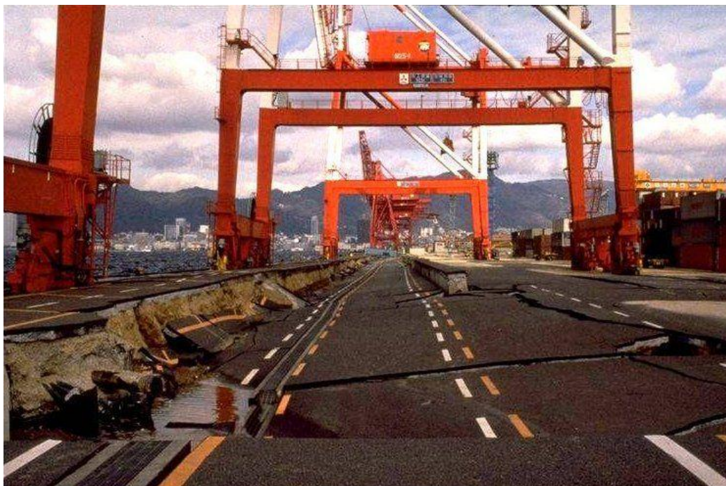
Figure 2.10: Liquefaction damage to man-made port islands in Kobe, Japan, after the 1995 Hyogo-Ken Nanbu Earthquake (Johnson 2000b)
