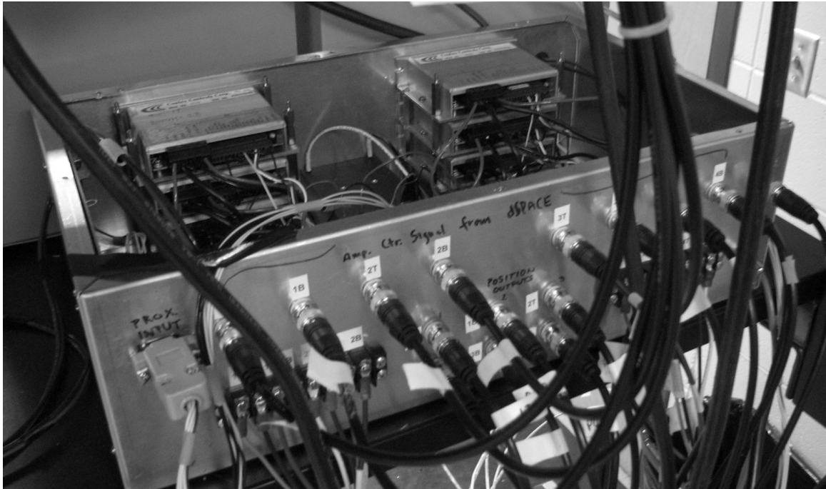
Figure 6-4 – Project Box for Active Magnetic Bearing Rig
