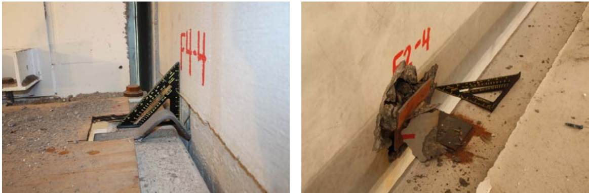
Fig. 3.35. Local failures examples along second floor support
