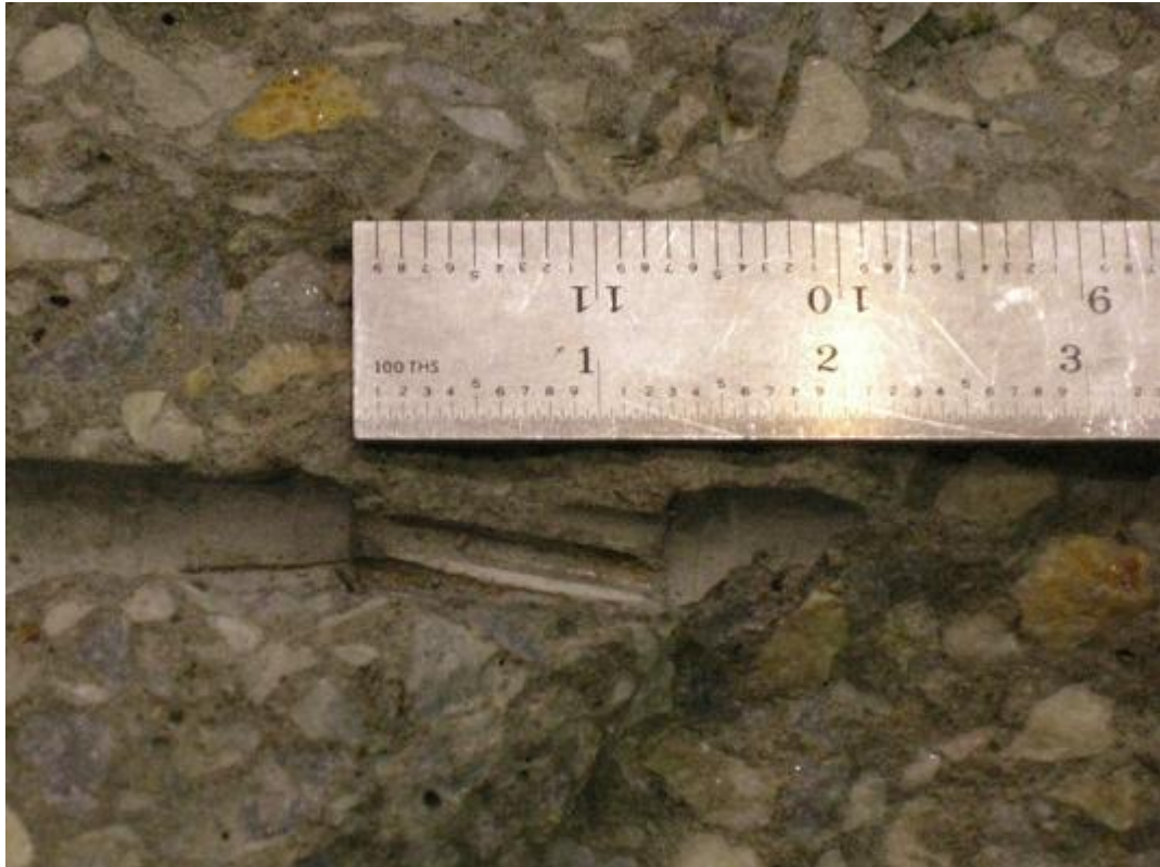
Figure 3.17: Unwinding failure of seven-wire strand during trial testing
