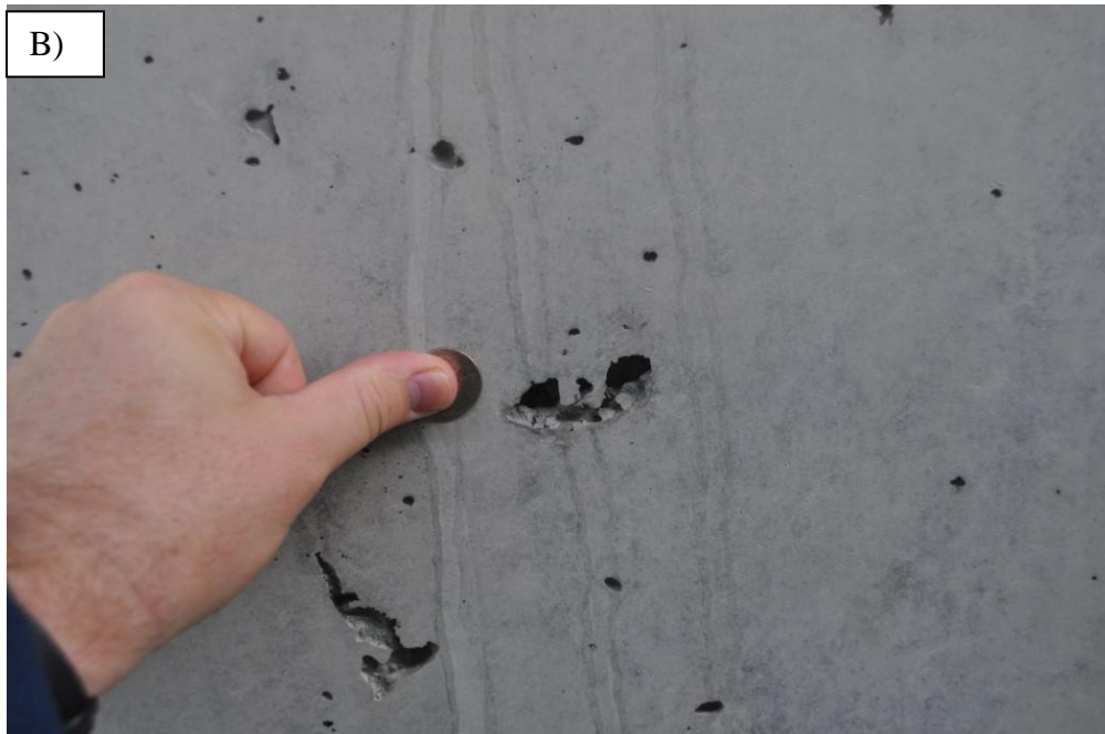
Figure 1.2: A) Typical surface finish achieved when using conventional concrete to produce precast, prestressed bulb-tees, and B) a bug hole in the beam surface
