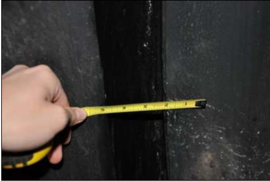
Figure 4-19: Joint Opening in HDPE Pipe
