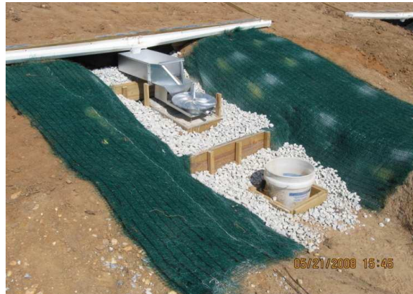
Figure 3.7. Newly installed gutter system, Coshocton wheel, and 20L sampling bucket for runoff sampling in 2008 at EVSRC (Baharanyi, 2010).
