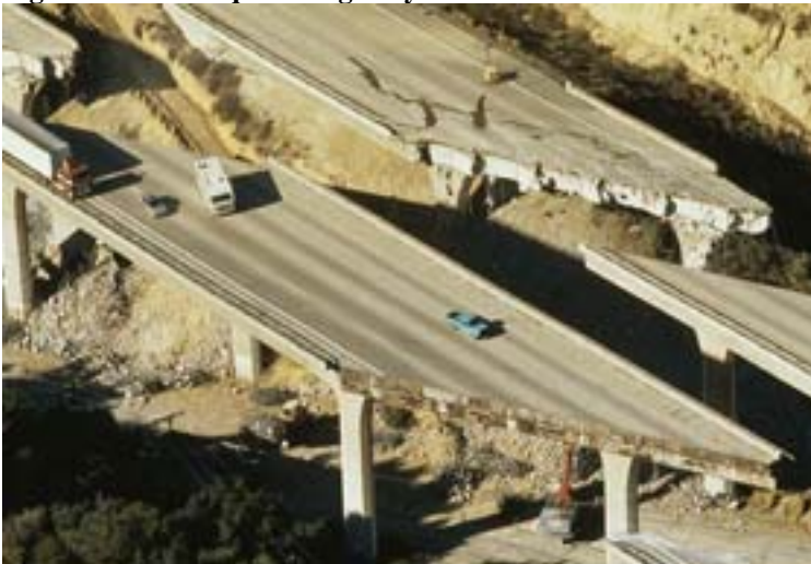
Figure 2.41 Earthquake Highway Destruction
