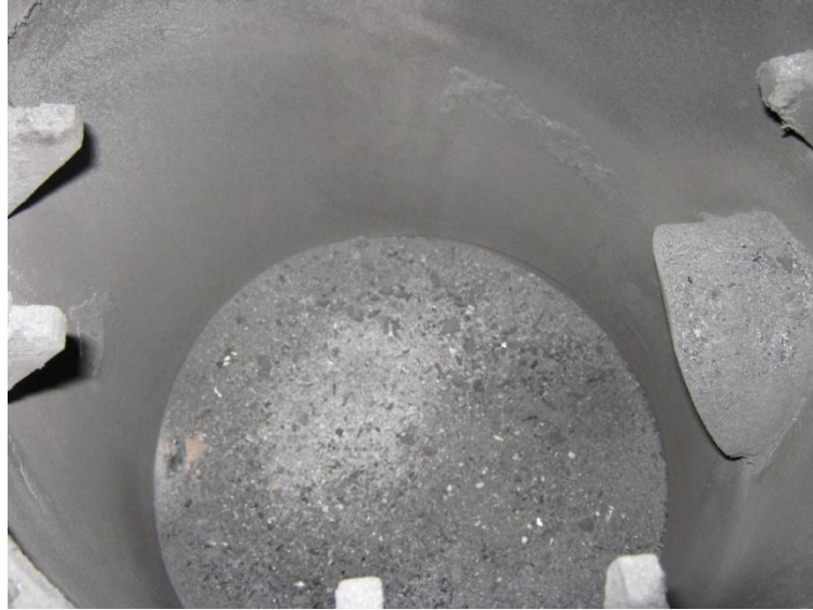
Figure 3.7: Chamber below grate, slanted entrance to tube leading to heat exchanger at right. Larger, heavier ash particles settle here
