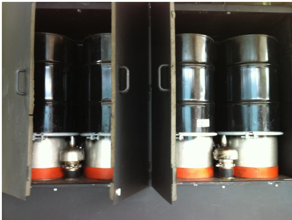
Figure 3.10: Filter box with doors open. Bags are inverted inside barrels by syngas flow
