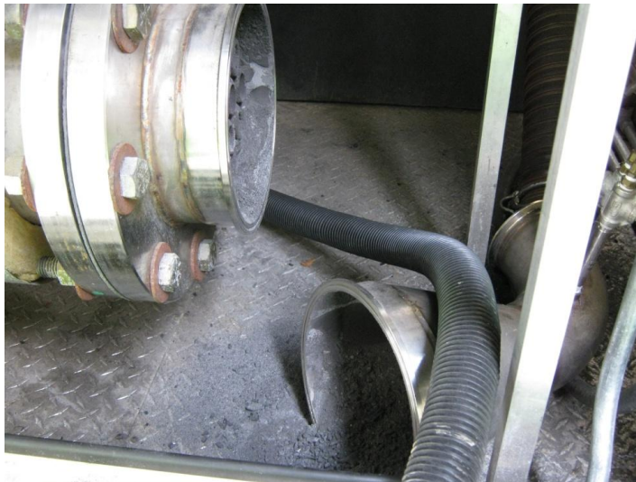
Figure 3.9: Heat exchanger exit, tubes visible inside at left. Pipe bend and flexible hose leading to filter box at right.
