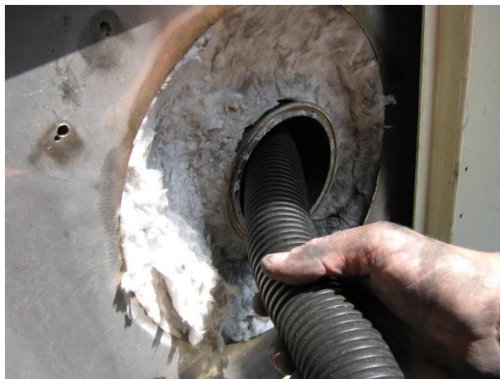
Figure 3.8: Access port at heat exchanger entrance, Shop-Vac in use
