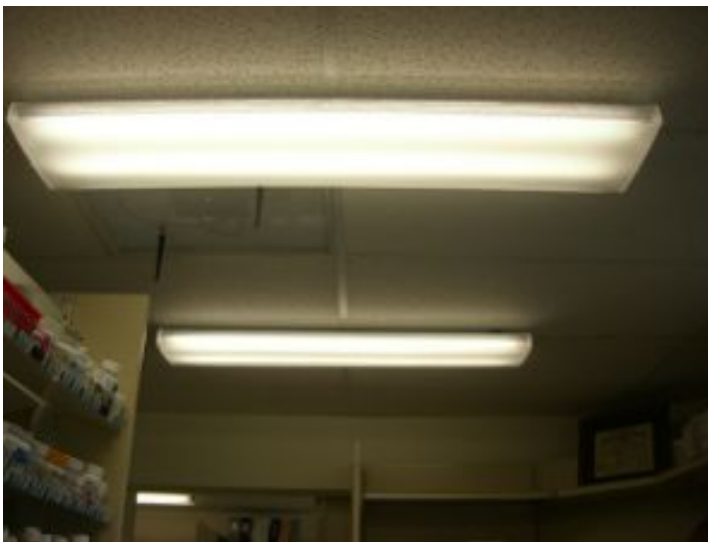
Figure 15: Light fixtures used in the pharmacy
