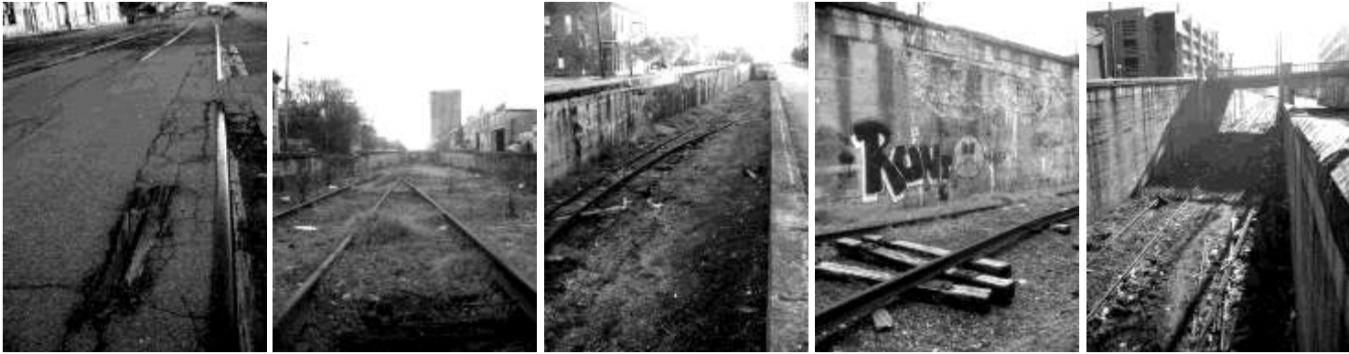
The above photographs reveal the present desolate conditions of the 1st Avenue South channel. (Photographs courtesy of the author.)
