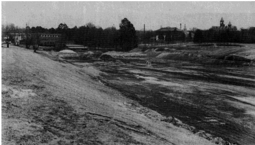
Figure 42: Land needed to be cleared and a stream filled in with dirt before construction could begin on Auburn Stadium. Circa 1937.
