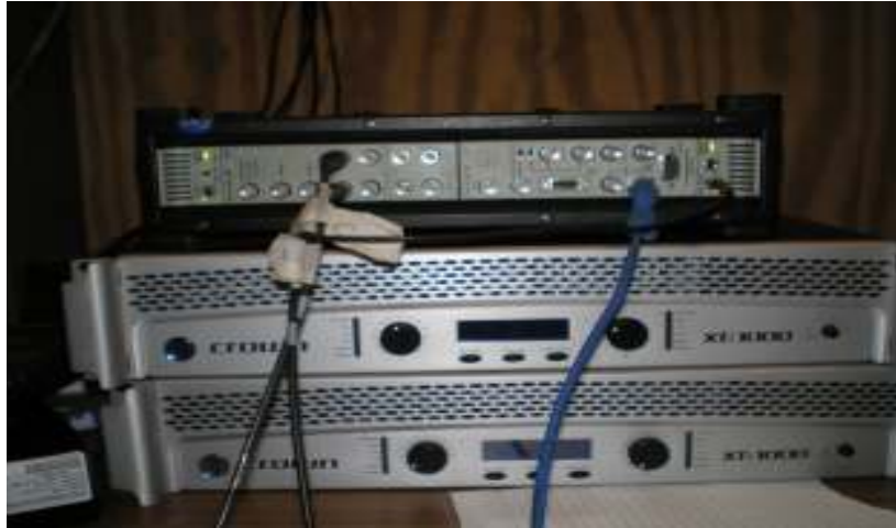
Figure 4.7: Brüel & Kjaer type 2827-002 on top of Crown XTi-1000 amplifiers
