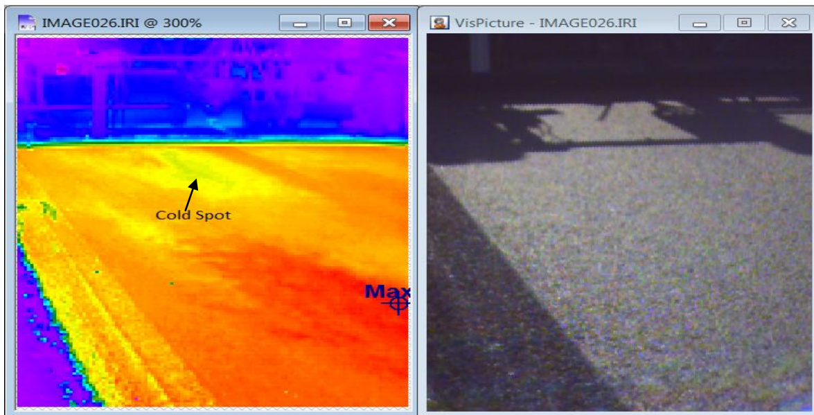
Figure 2.3: Cold Spot (Infrared Image taken from I-R Analysis Software)
