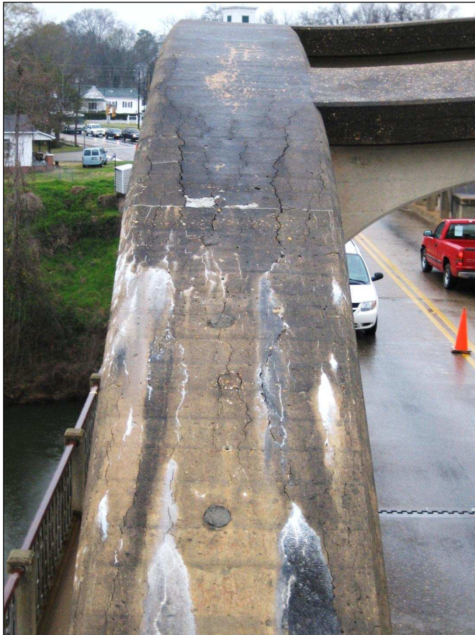
Figure 3.26: A closer view of the severe distress due to ASR on the eastern side of the southern arch of span 5 on 3-11-2008
