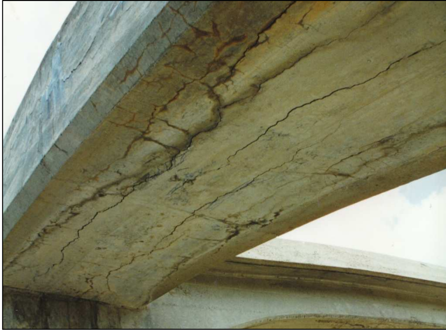
Figure 3.29: Severe cracks on the bottom of the arch on 3-11-2008
