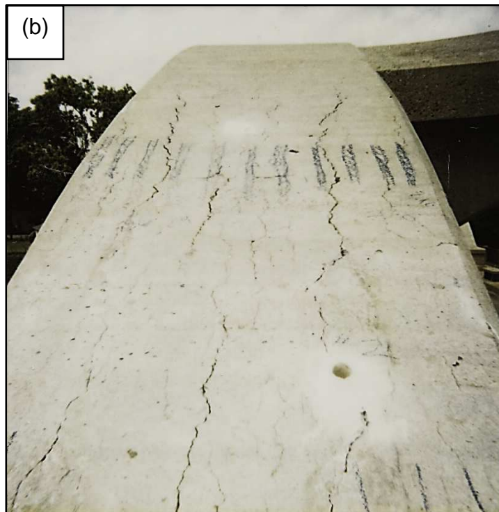
Figure 3.9: Examples of distress in the late 1990s on the a) top and b) bottom of a span 5 arch
