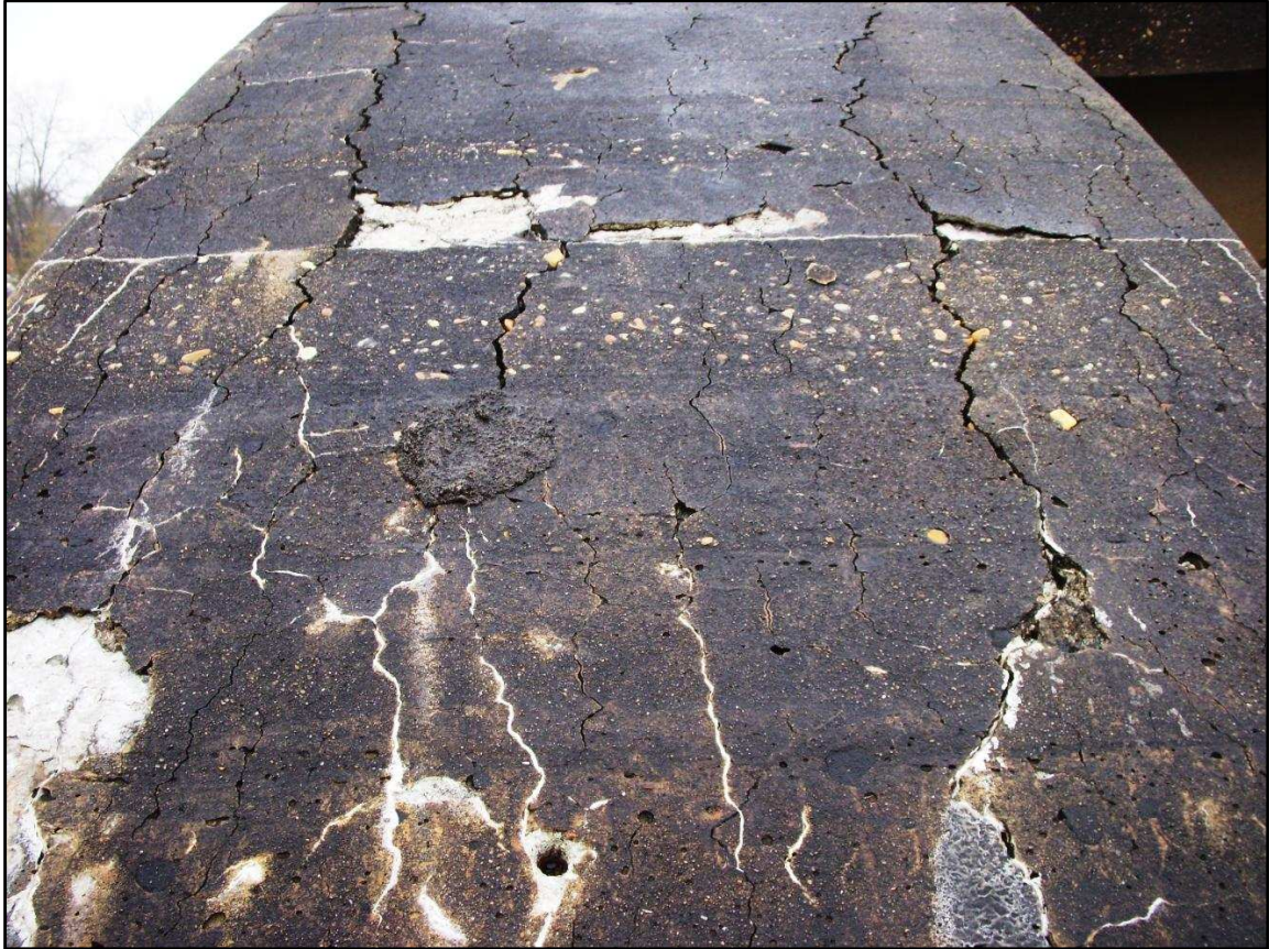
Figure 1.2: ASR-Induced cracking on the Bibb Graves Bridge
