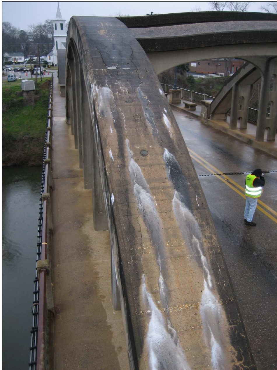
Figure 3.25: Severe distress due to ASR on the eastern side of the southern arch of span 5 on 3-11-2008
