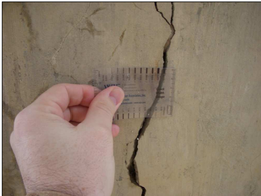
Figure 3.28: Severe cracks greater than 0.1 inches on 3-11-2008
