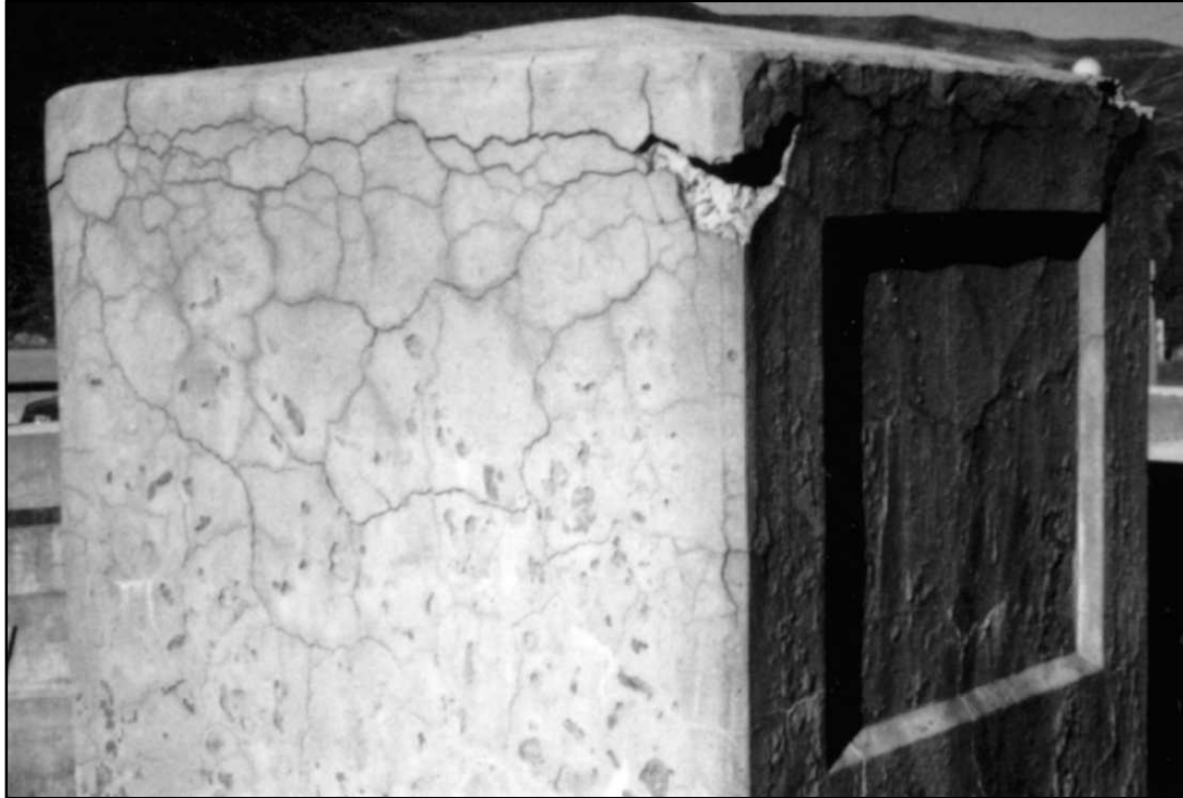
Figure 2.5: Typical “map-cracking” due to ASR (Forster et al. 1998)
