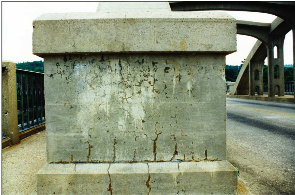
Figure 3.30: Map-cracking on the abutment of span 5
