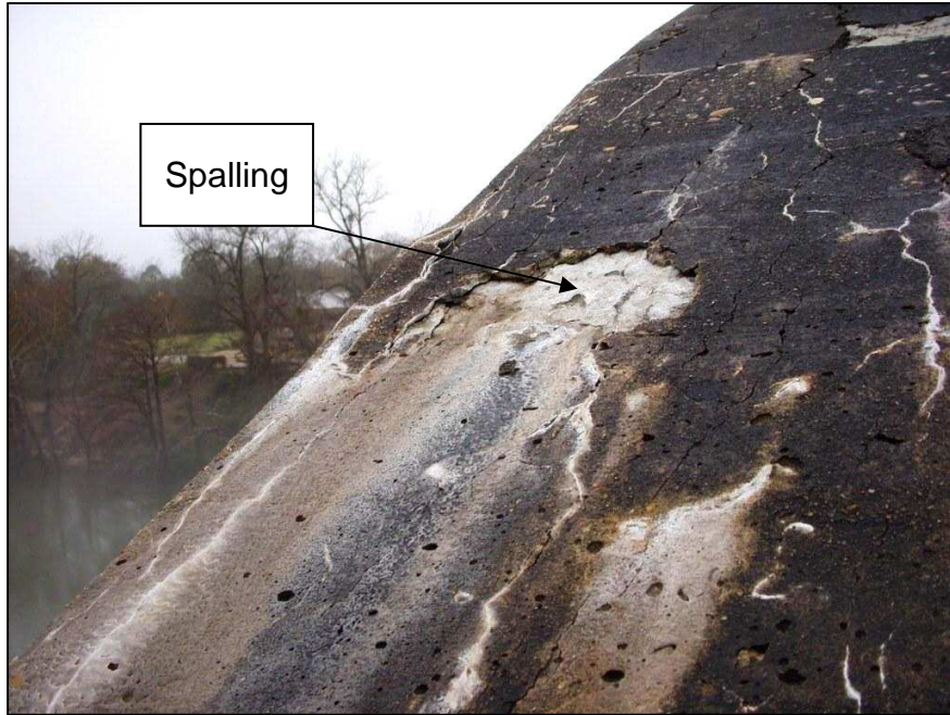
Figure 3.27: An example of spalling on span 5 on 12-14-2009
