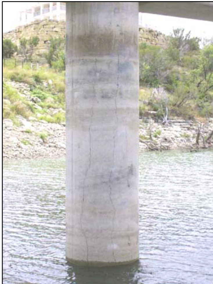
Figure 2.10: ASR-cracking orienting itself to underlying steel reinforcement
