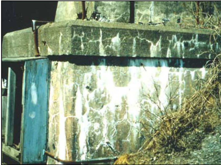
Figure 2.13: Example of efflorescence and alkali-silica gel exuding to the surface of a concrete foundation suffering from ASR (Fournier et al. 2004)
