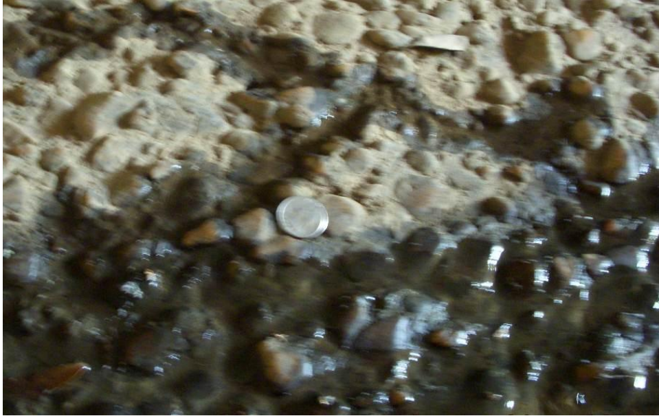
Figure 3-43: Base Deterioration in Prattville Culvert on US-82
