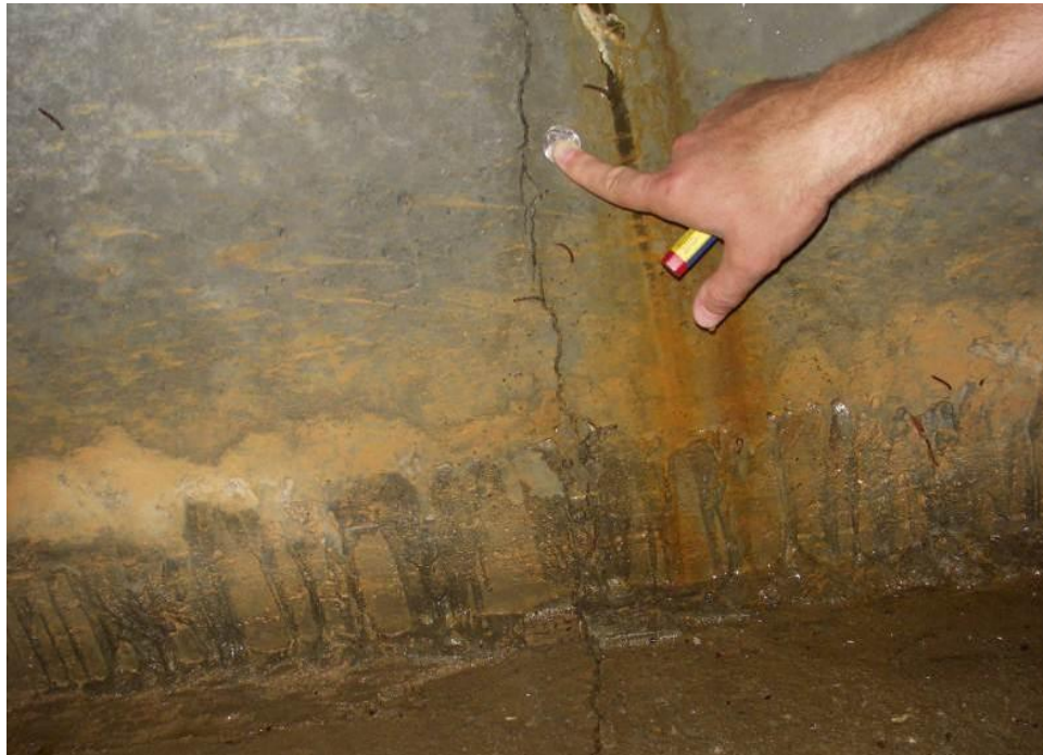
Figure 3-9: Transverse Wall and Base Crack in AEB Culvert at 175+70 that is greater than 0.08 in. (2 mm) wide
