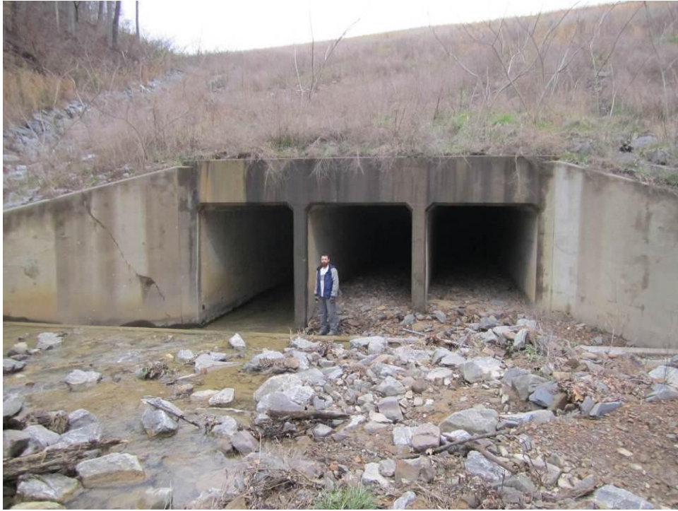
Figure 3-27: Corridor X Culvert at 4959+43 Entrance and Wingwall Crack
