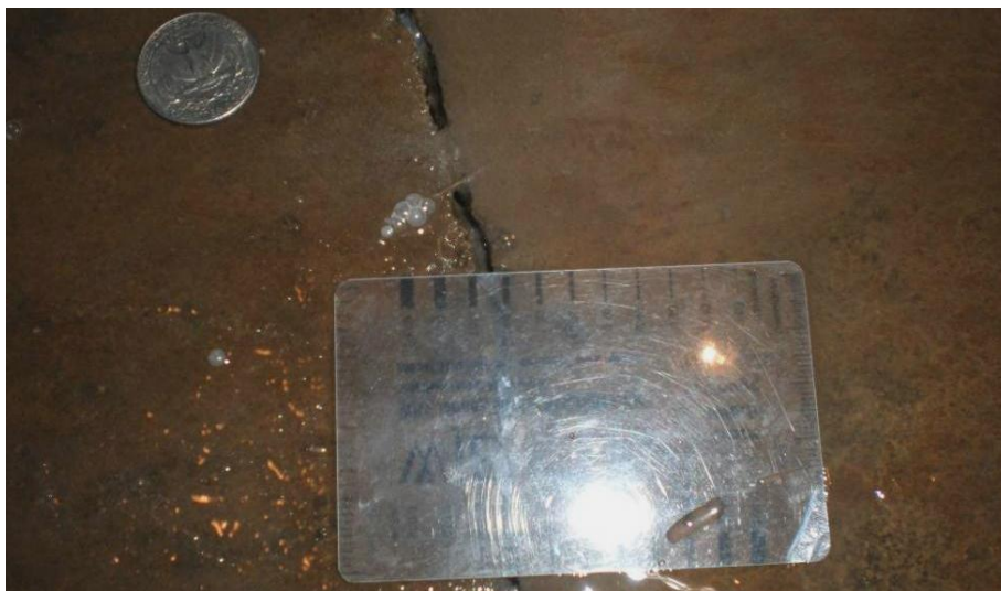
Figure 3-11: Base Crack from AEB Culvert at 240+37
