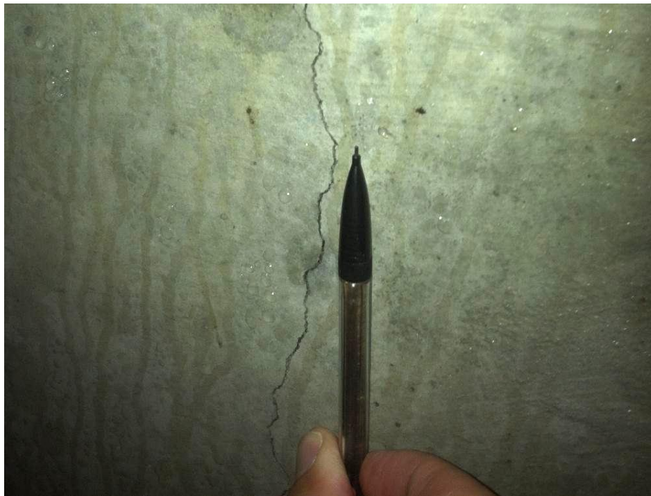
Figure 3-31: Transverse Wall Crack in Corridor X Culvert at Exit 85
