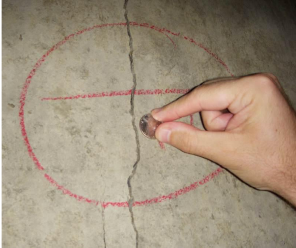
Figure 3-4: 1/4 in. (6.4 mm) Wide Transverse Crack in AEB Culvert at 149+60 at Station 308 ft 0 in. in the North Wall
