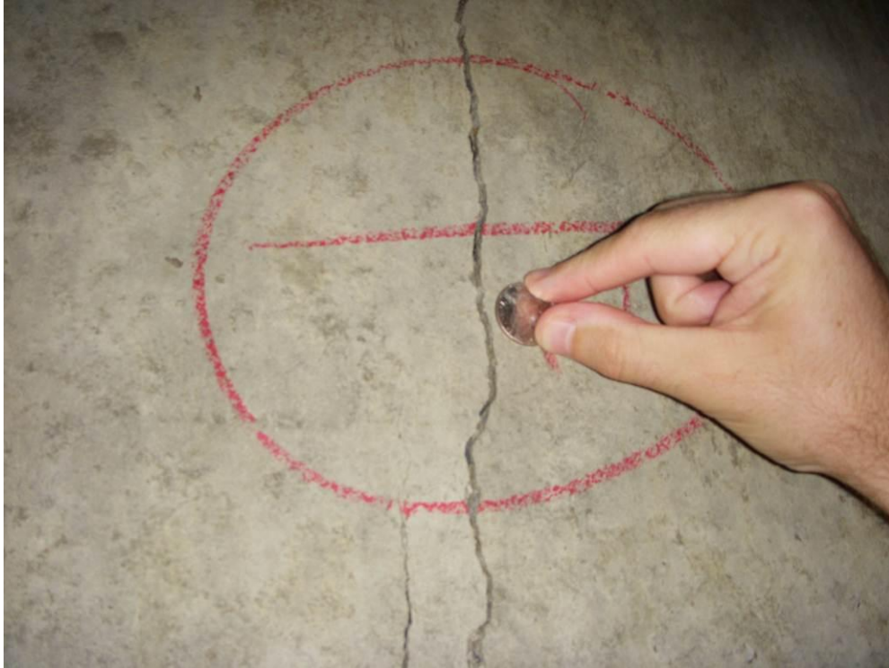
Figure 2-1: Through Crack in a Culvert in the Anniston East Bypass (AEB) Project (149+60)
