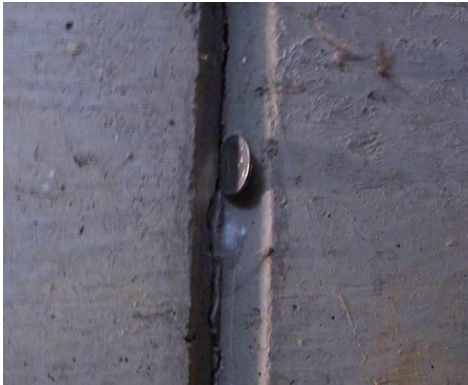
Figure 3-47: Crack in the Vee Joint in the Wall in I-85 South Culvert
