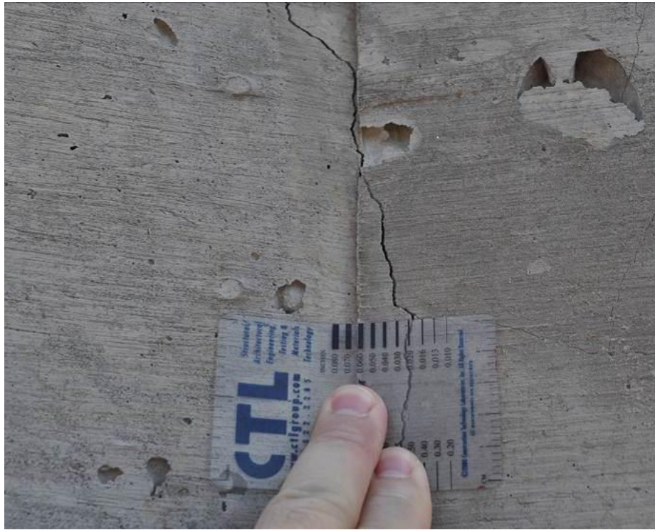
Figure 3-20: Crack at Wingwall and Culvert Intersection in Centreville Culvert at 1808+98
