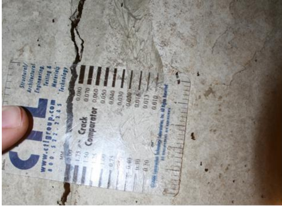
Figure 1-1: Transverse Crack in the AEB Project (Crack Width \approx 0.08 in. [2 mm])
