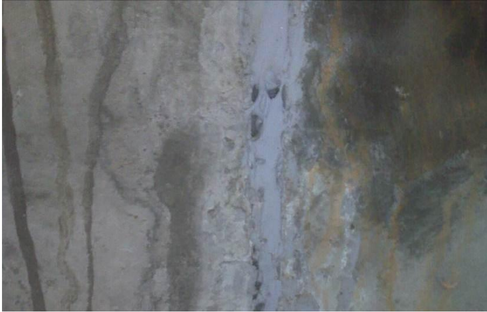
Figure 3-25: Transverse Contraction Joint in the Exterior Wall of Corridor X Culvert at 4877+13 at Station 341 ft 3 in.
