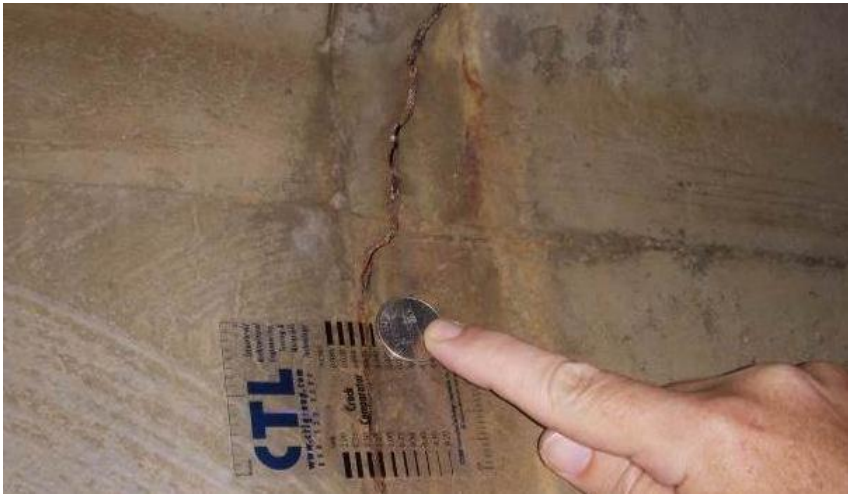
Figure 3-40: Transverse Crack in South Wall at Station 110 ft 11 in. of Dutton Culvert at 548+23 that is Greater than 1/4 in. (6.4 mm) Wide
