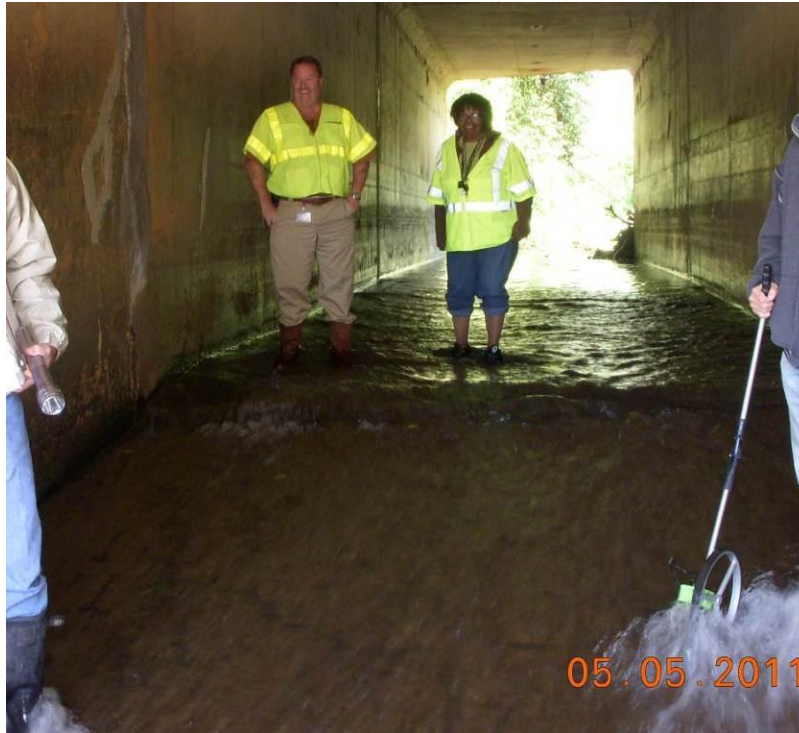
Figure 3-42: Settlement of Prattville Culvert on US-82
