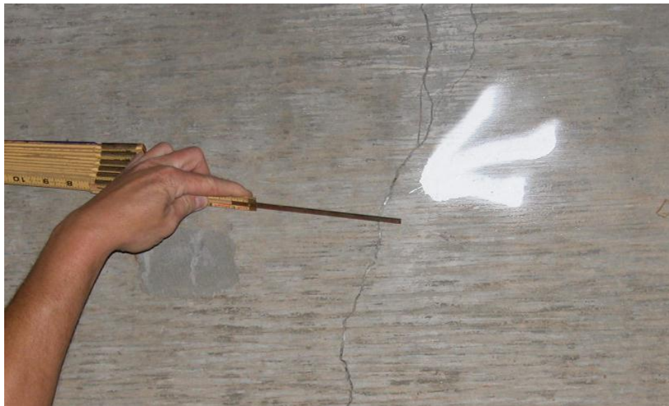
Figure 3-35: Transverse Wall Crack in Dadeville Culvert at 45+31.55
