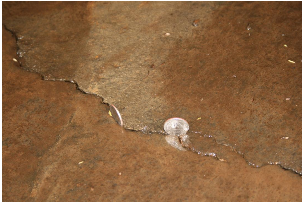
Figure 1-2: Transverse Base Crack in the AEB Project (Crack Width > 0.06 in. [2 mm])
