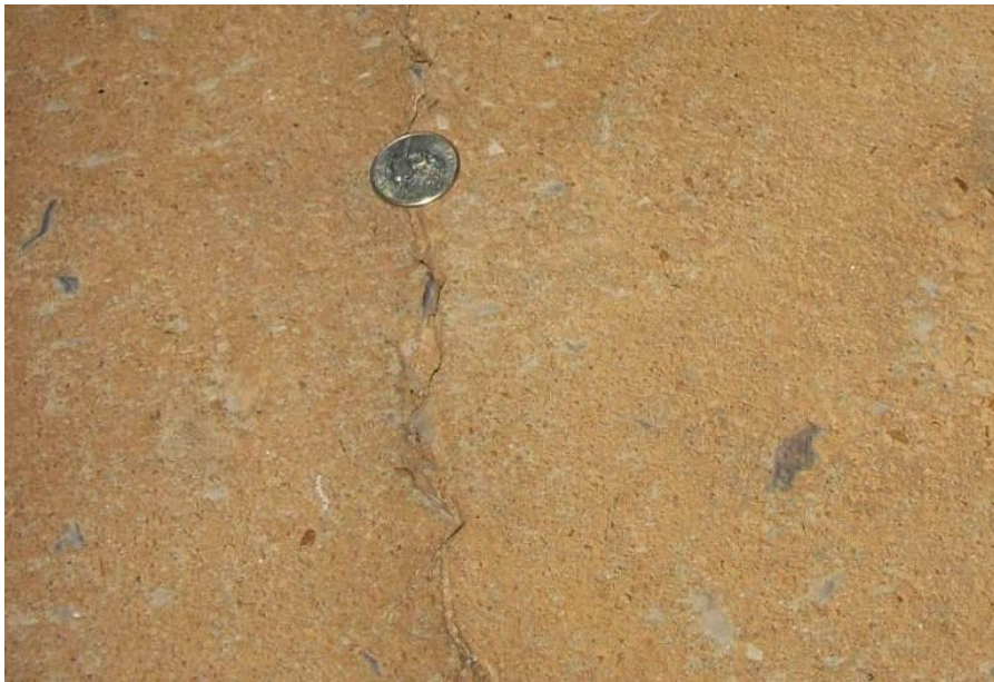
Figure 3-6: 1/4 in. (3.2 mm) Wide Transverse Base Crack at Station 179 ft 0 in. in AEB Culvert at 162+90
