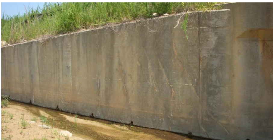
Figure 3-12: Wingwall Cracks in AEB Culvert at 240+37
