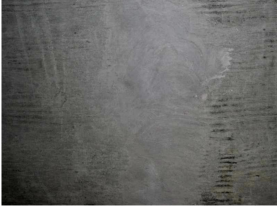
Figure 3-19: East Barrel Wall Crack Covered with Mortar in Centreville Culvert at 1808+98
