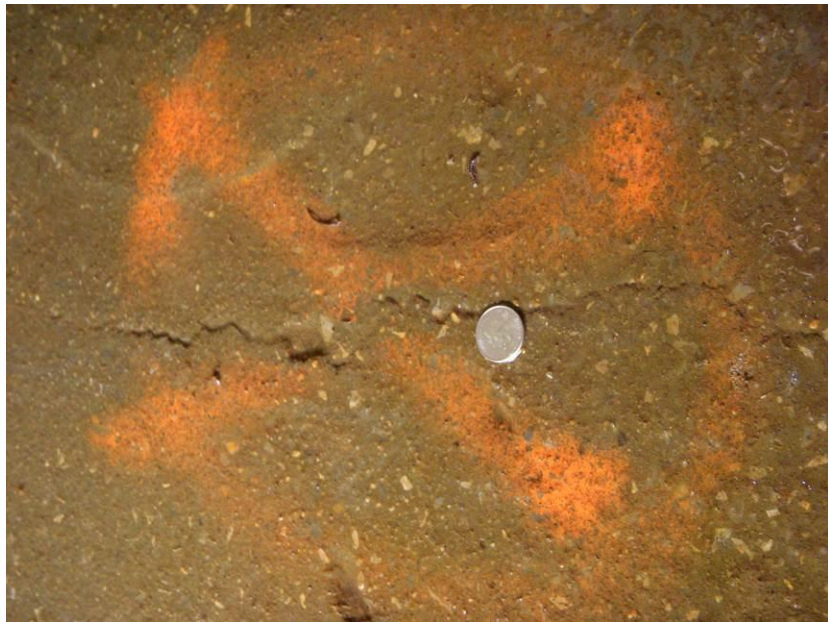
Figure 2-6: Plastic Shrinkage Crack in the Anniston East Bypass Project (175+70)
