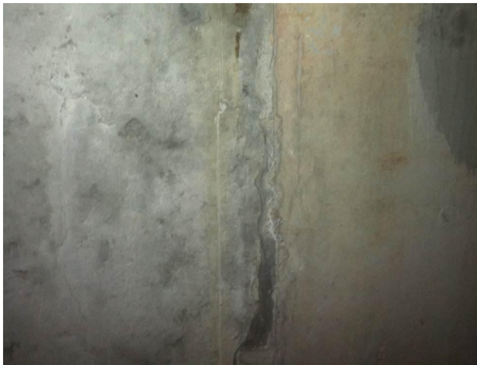
Figure 3-32: Transverse Construction Joint in Corridor X Culvert at Exit 85 (Joint Patched with Mortar)
