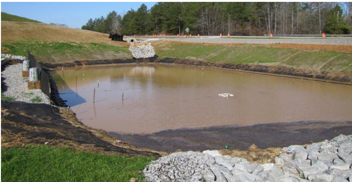
Figure 6.2: Stormwater overtops the baffles when the basin fills to capacity.
