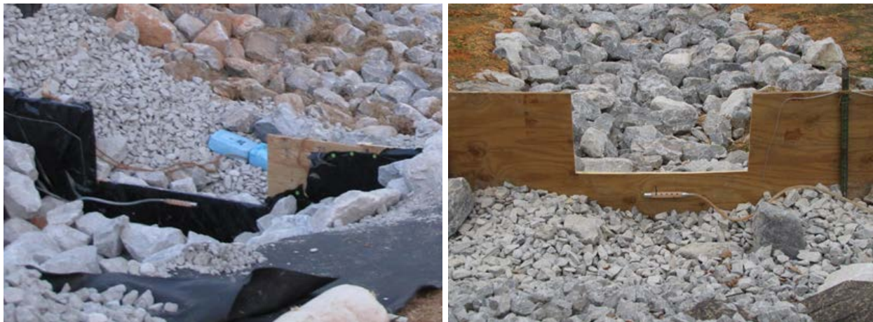
Figure 4.7: Bubbler tube and suction head installed on primary/secondary inflow channels.
