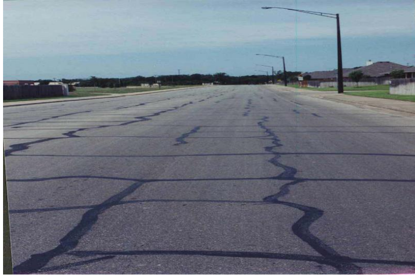
Figure 2.5: Reflective Cracking from excessive shrinkage of base layer (Scullion 2002)
