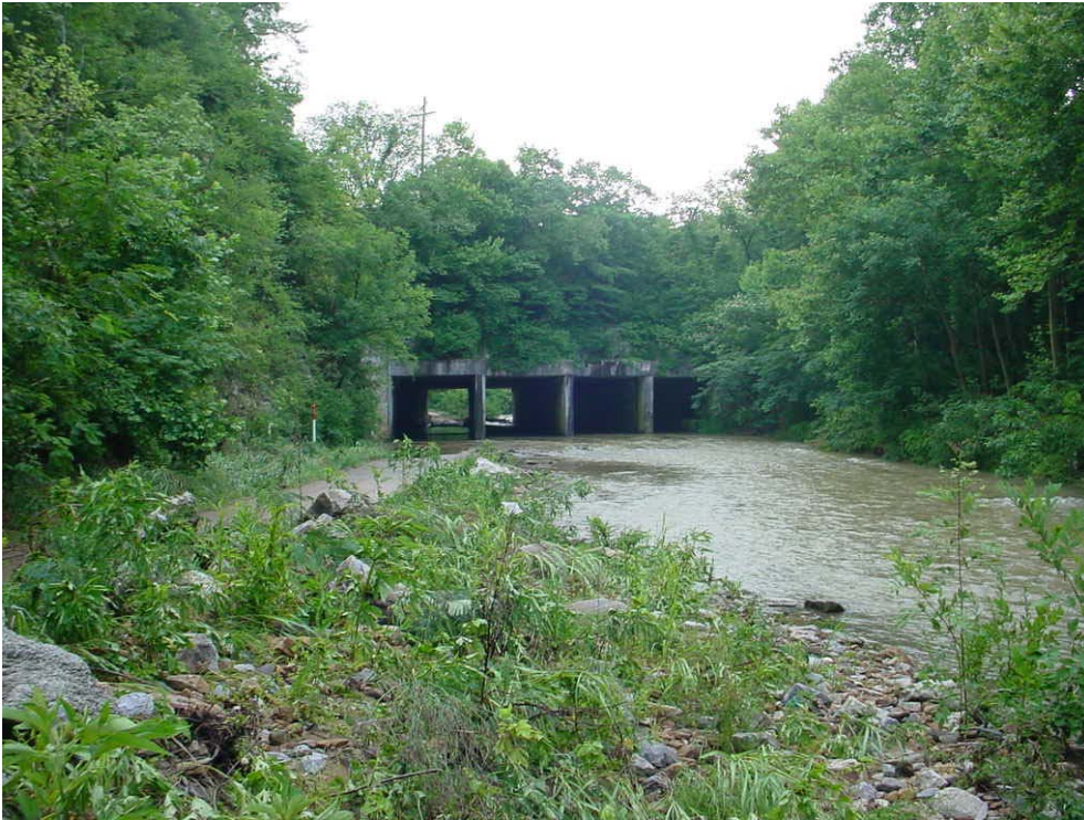
Figure 29. Section A, outlet of the box culvert at the L and N Railroad.
