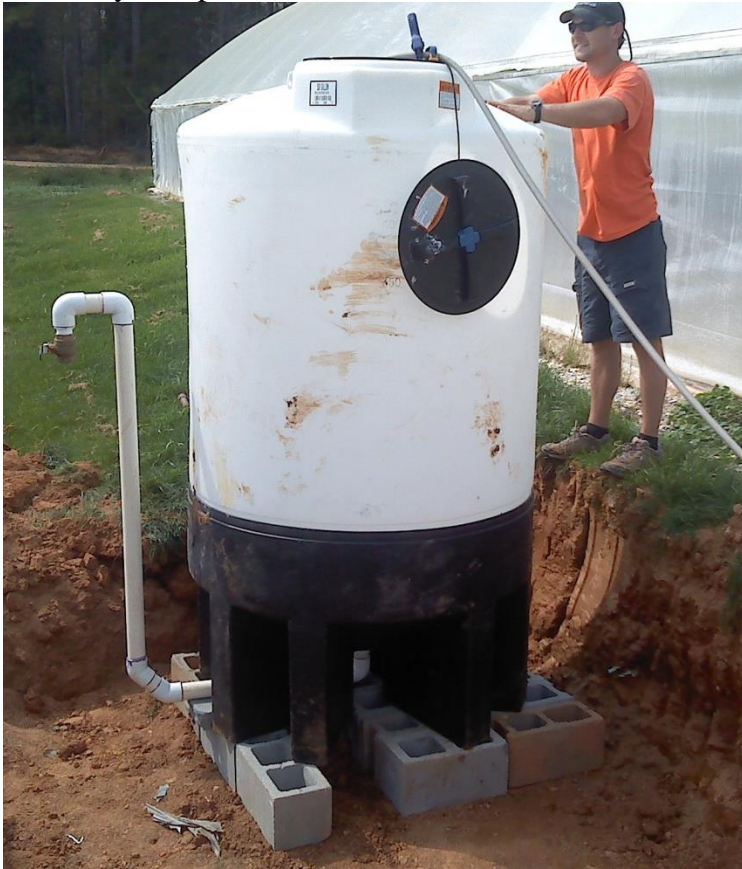
Figure 14A. Installing the cone-bottom tank (i.e. clarifier) used to treat the biofloc system production water.
