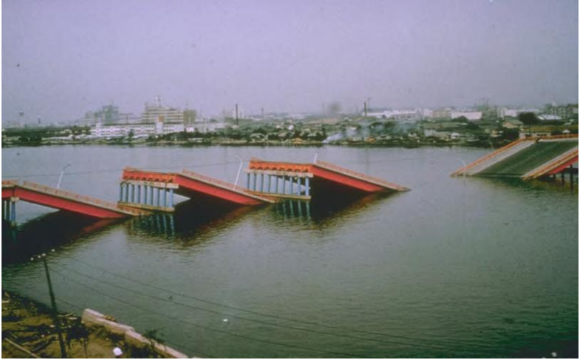
Figure 2.4. Collapse of the showa bridge in the 1964 Niigata, Japan earthquake (NGDC as referenced in Kavazanjian et al. 2011)
