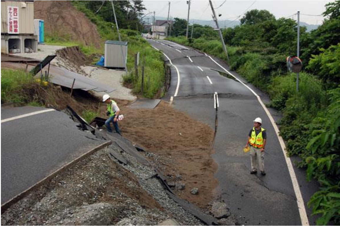
Figure 2.3. Flow liquefaction damage to a road in Japan during an offshore earthquake in 2007 (USGS, 2008)
