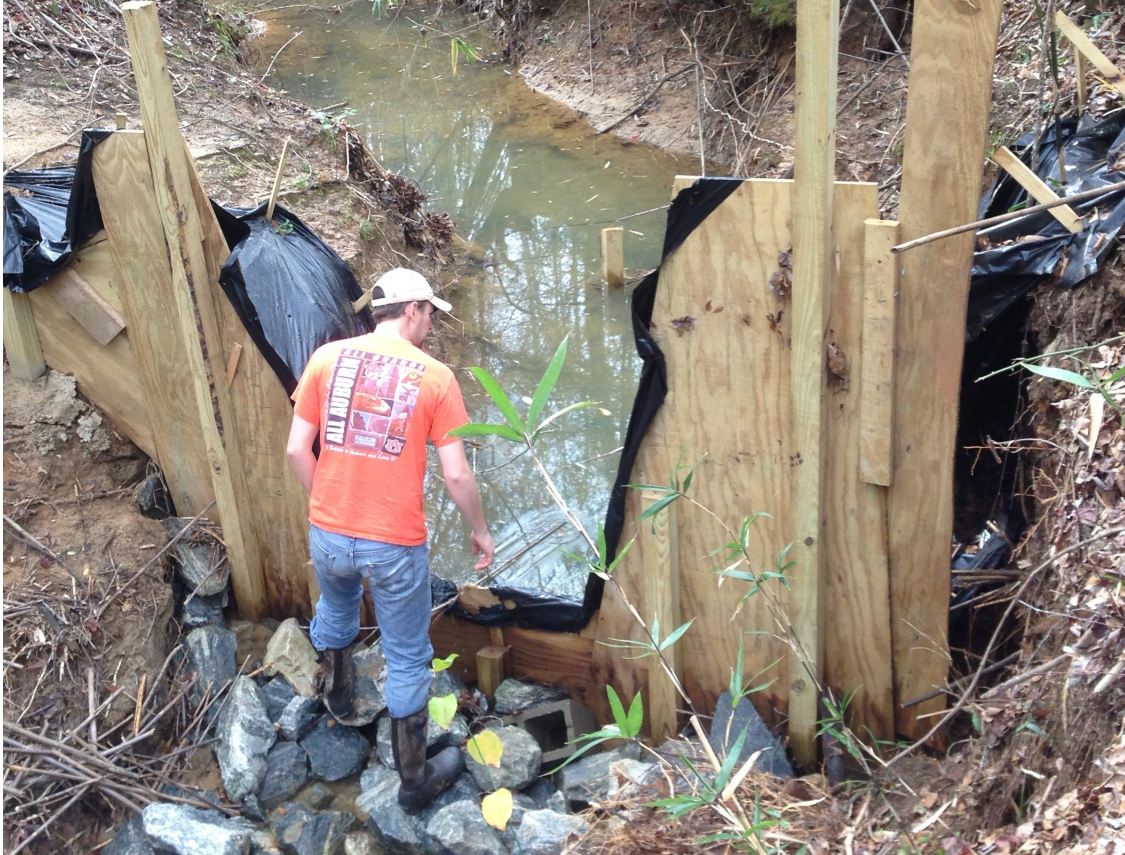
Figure 3.17: Erosion damage at the Cipolletti weir to the right
