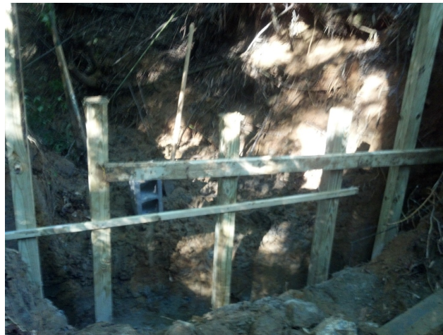
Figure 3.7: Support post for the Cipolletti weir
