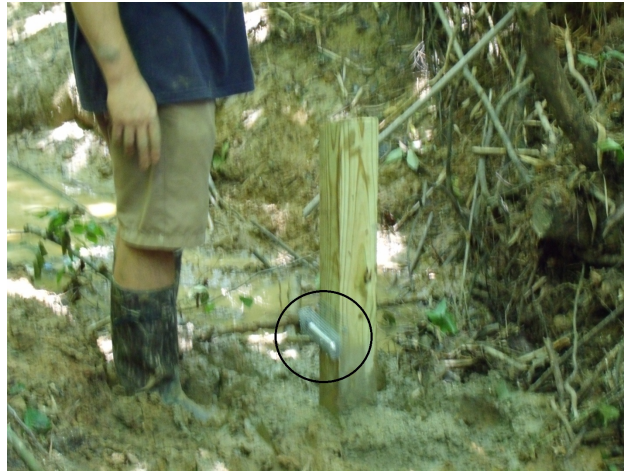
Figure 3.16: HOBOT pressure sensor installed upstream at each weir
