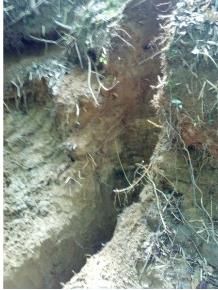
Figure 3.6: Roots causing issues on the lateral walls of the weir
