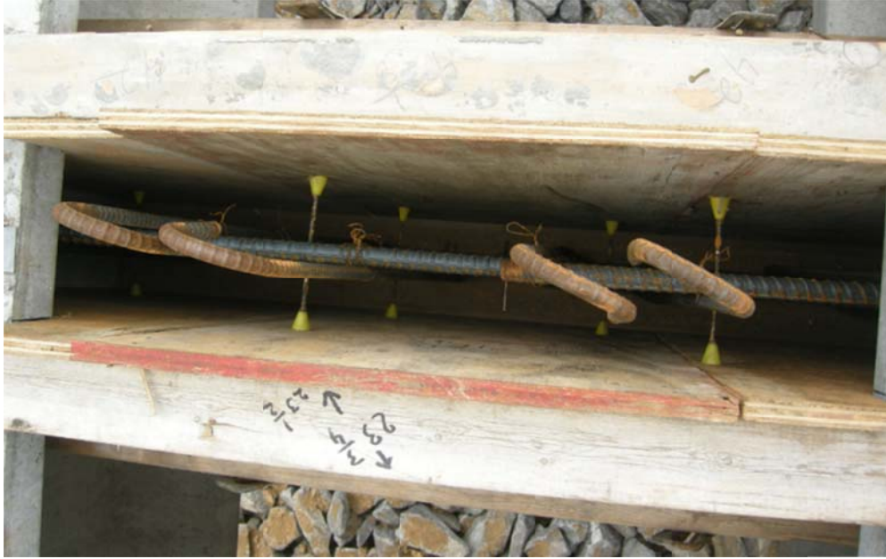
Figure 3.17. A view from above the rebar and form of a webwall between two VC BT-54s.
