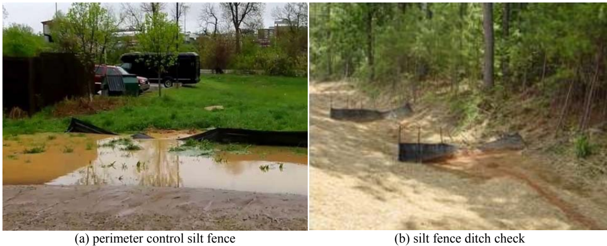
Figure 6.12: Silt Fence Structural Failures.
