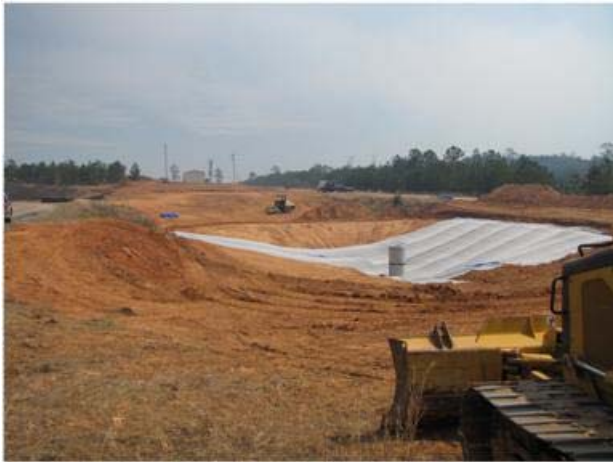
(c) liner rolled out after the first day of pond liner installation
