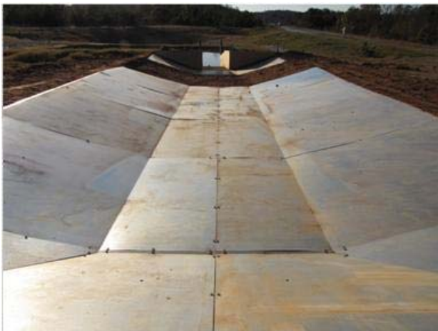
(e) view of the channel liner from the top of the channel
