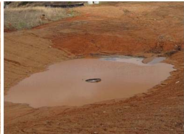
(b) ponding around temporary riser
