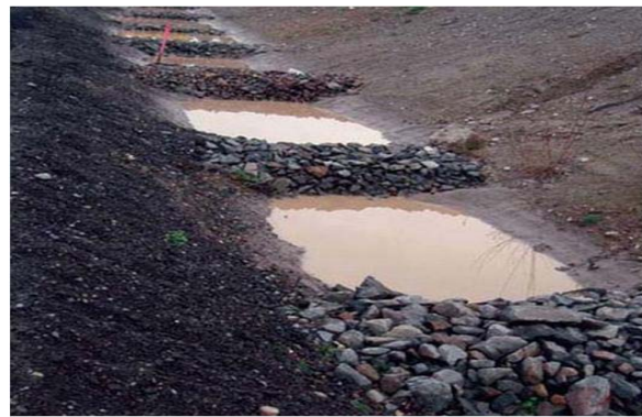
(b) rock ditch checks detaining water
