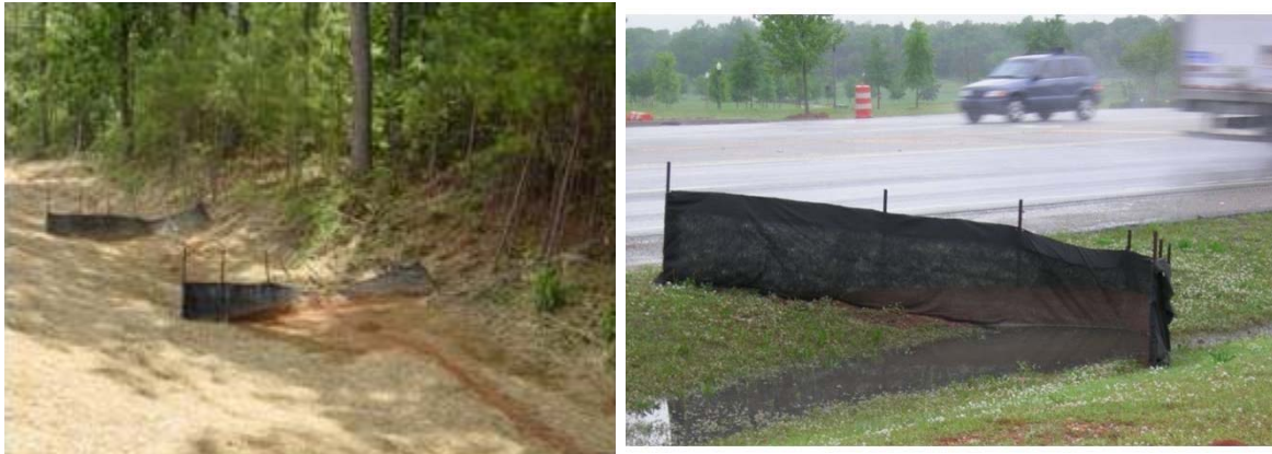
(a) improperly maintained silt fence ditch check (b) properly maintained silt fence ditch check
