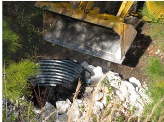
(b) riprap placed around riser pipe for support during ponding periods
