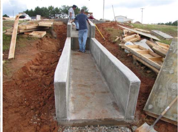
(d) constructed conveyance channels
