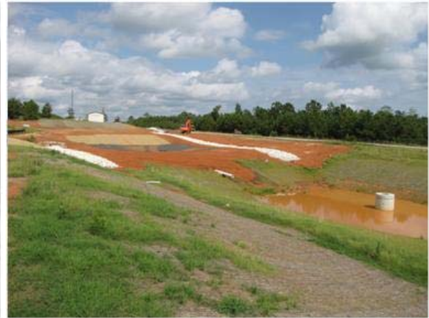
(d) overall view of the facility after installation of the drainage channels
