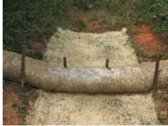
(b) straw wattle w/PAM dosing check dam
