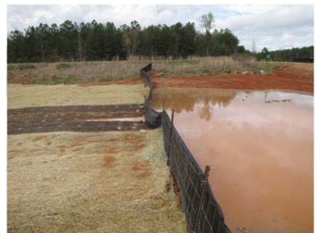
(b) TRM conveying impounded runoff
