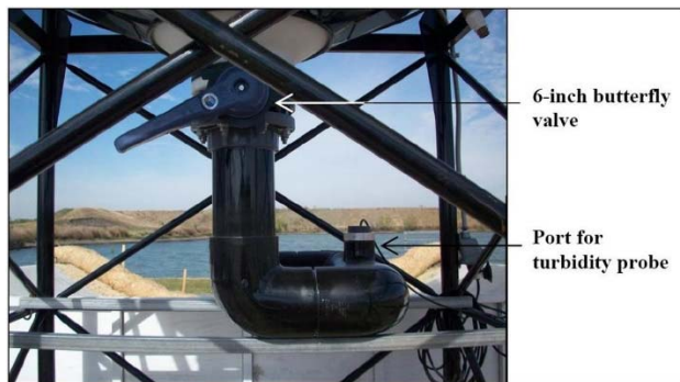
(b) mixing tank release valve and turbidity meter
