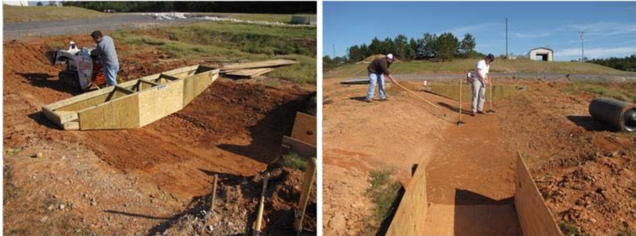
(a) trapezoidal mold used for fine grading of the channel (b) fine grading to achieve the desired channel shape
