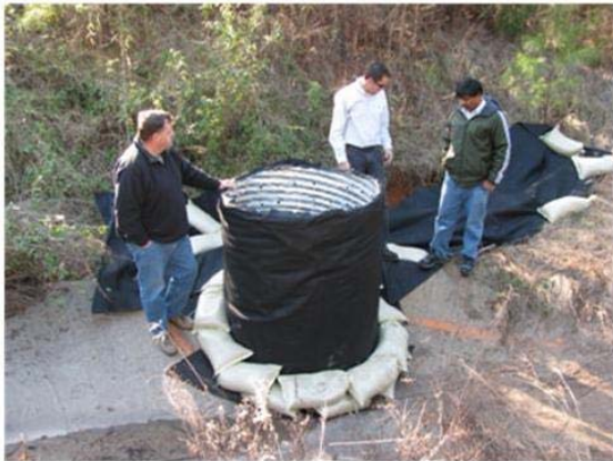
(a) perforated riser pipe wrapped in filter fabric with a wire trash guard
