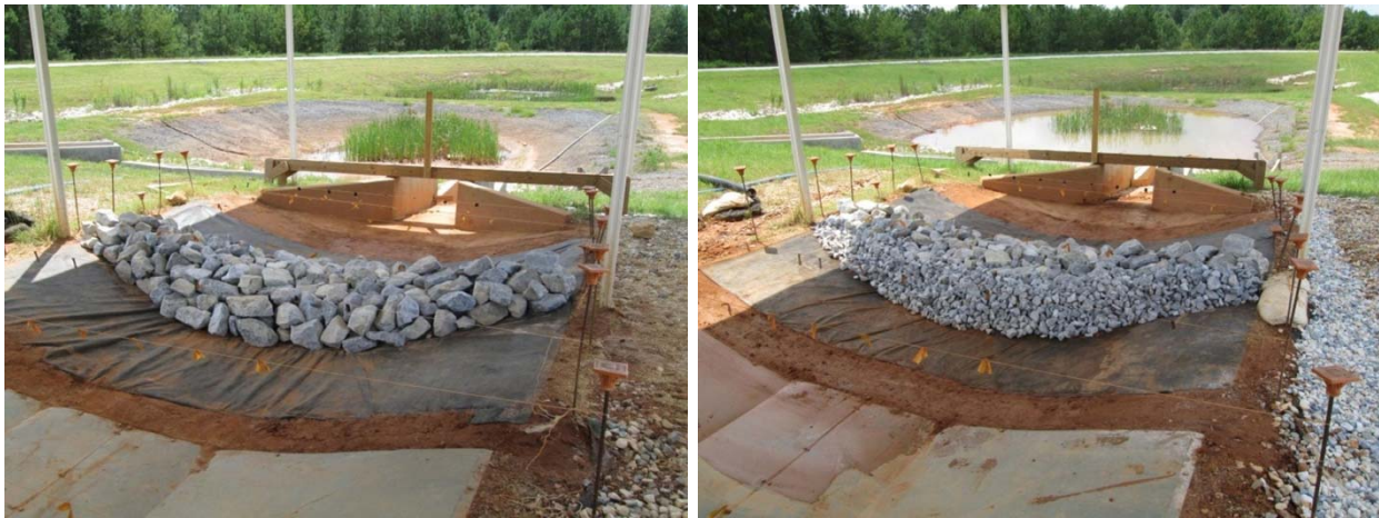
(a) Riprap ditch check w/no choker
