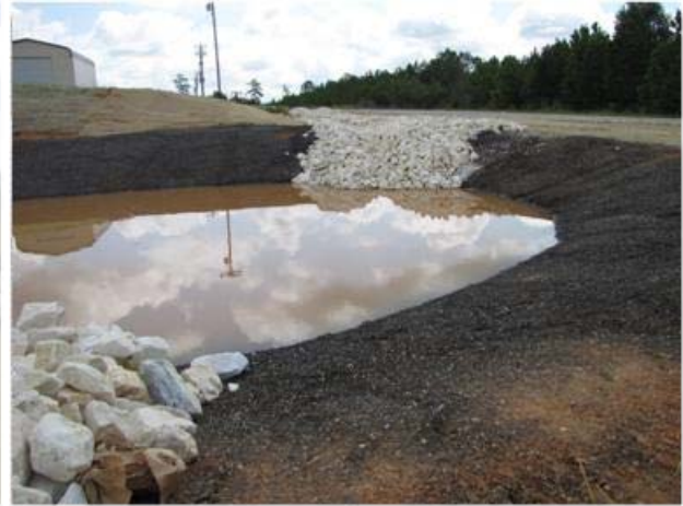
(b) inlet channel responsible for conveying runoff from the parking lot to the pond
