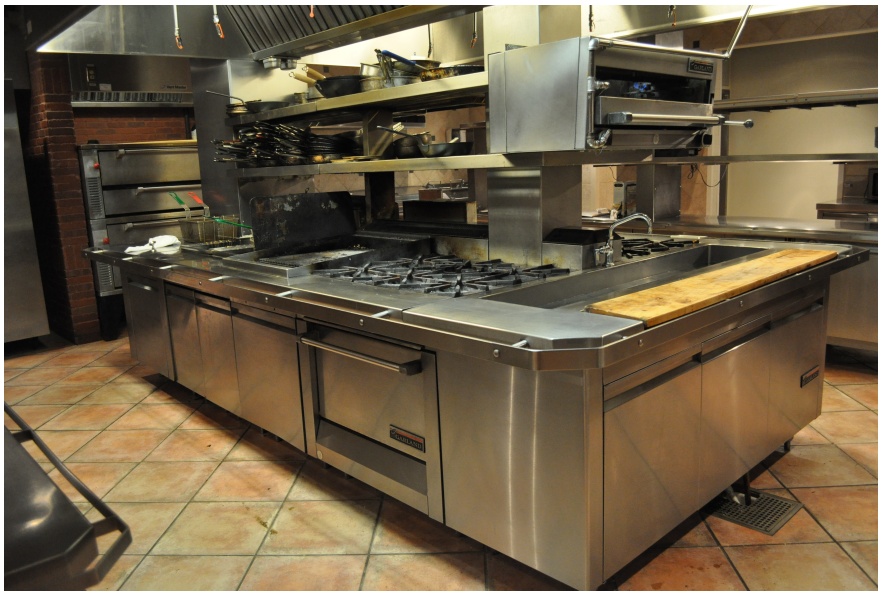
Figure 2: Photo of double cook line in restaurant kitchen
