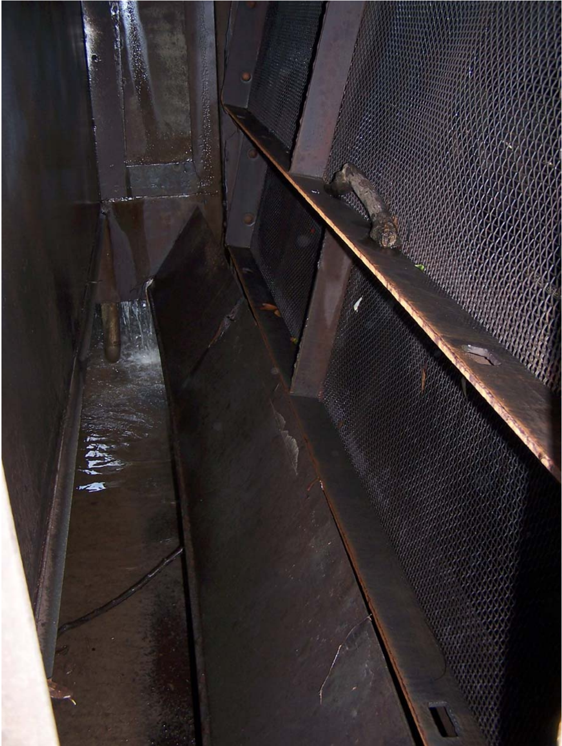
FIGURE 40. – Example of cooling water intake structure screen ledge for Barry, Gadsden, E.C. Gaston, Gorgas, and Greene County Steam Plants during 316(b) sampling conducted by Alabama Power Company in 2004-2005.
