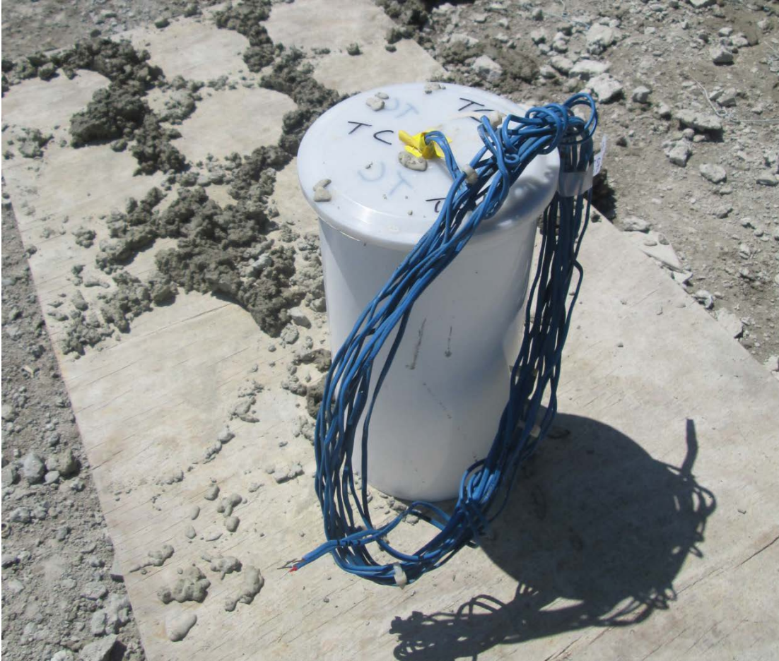
Figure 4.18: A Thermocouple Cylinder, Ready for Connection
