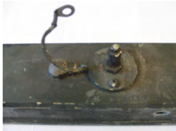
Figure 6.8: Example of an old style hard wire grounding apparatus
