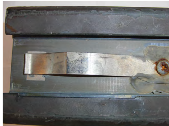
Figure 6.2: Example of wear on rail extrusion
