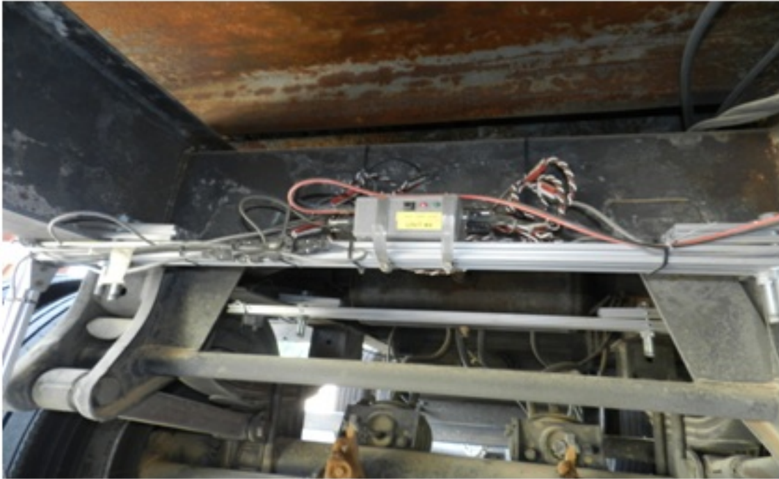
Figure 2.18: Mounted CAN Box
