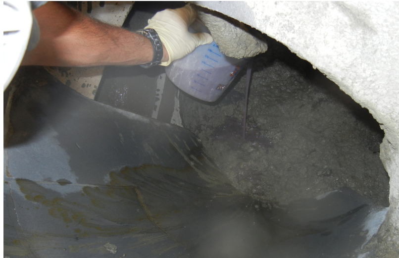
Figure 3-12: HRWRA being placed directly on to the concrete in the ready-mixed concrete truck
