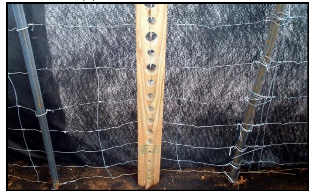
(f) MFE-I Dewatering Board
