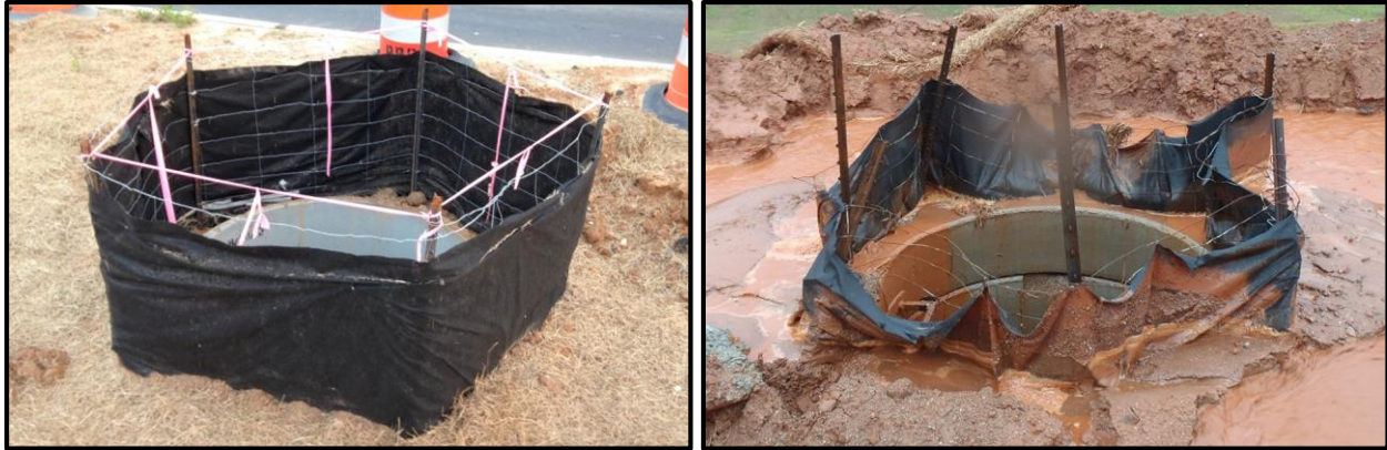
(a) typical installation on bare soil (b) improperly maintained installation Figure 2.3 Typical Silt Fence Inlet Protection Installation and Failure Mode.
