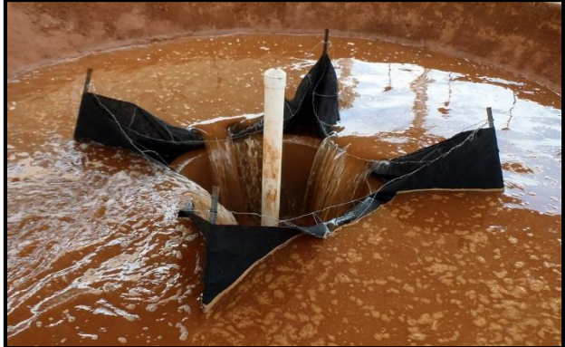
(b) Typical Installation Failure
