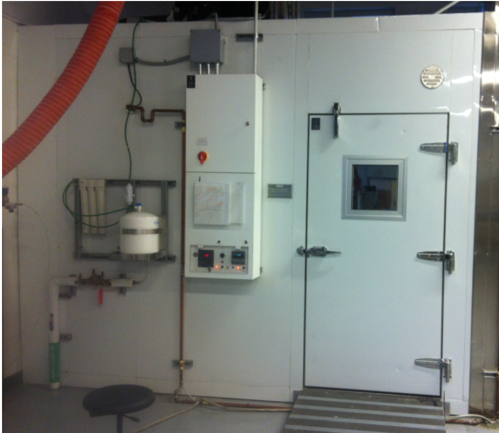
Figure B.5: Walk-in freezer for woodchips storage
