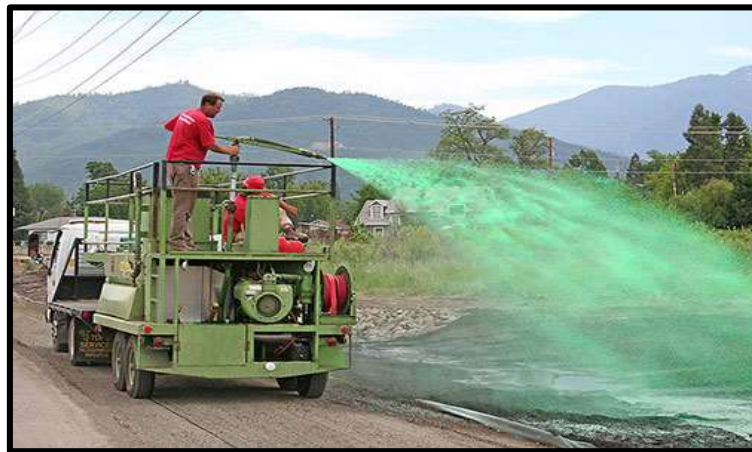
Figure 2.2: Hydra CX2 ® hydromulching operation in the field for erosion reduction (Source: www.fostersupply.com )
