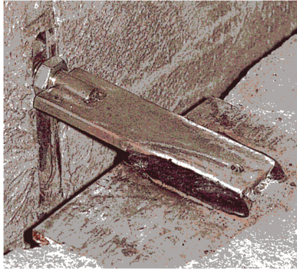
Figure 2-8 Slotted Strap PSA Connection Welded to a Slab Embed (Oswald and Bazan 2013)
