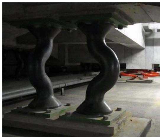
Figure 2-28. Lead Dampers (Front) and Helical Steel Dampers (Back) (Mori Living, 2011)
