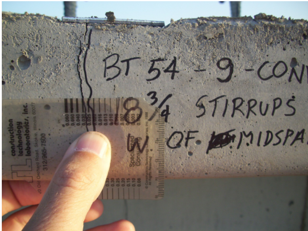
Figure 3-40: Crack Width in BT-54 Girder Prior to Prestress Transfer
