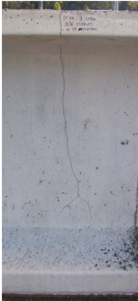
Figure 3-39: Crack in BT-54 Prior to Prestress Transfer
