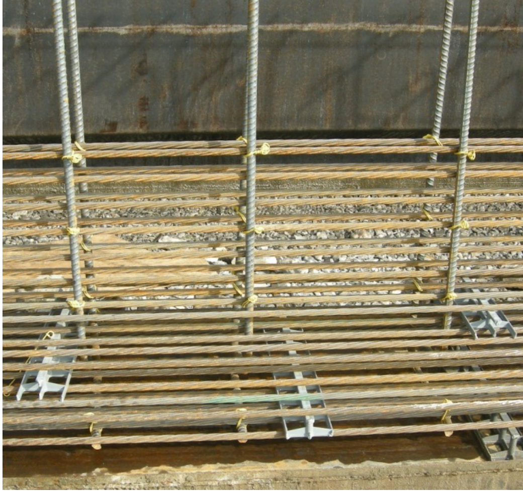
Figure 3-27: Prestressing Wire Surface Condition
