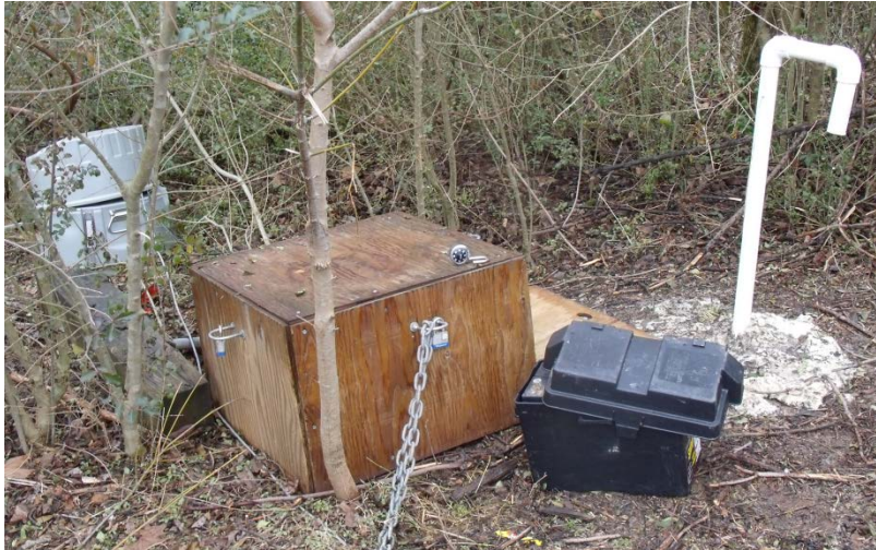
Figure 3.6: Installation of the groundwater well at the downstream site of the interstate; also picture is the auto sampler and the wooden box used to shelter the auto-sampler battery.
